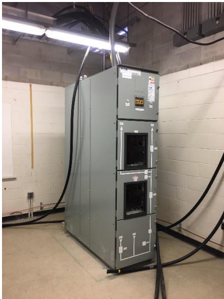
Lakehead - New PCT building switchgear
