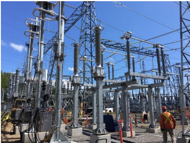
Lakehead – Ground switches in Bay 9
