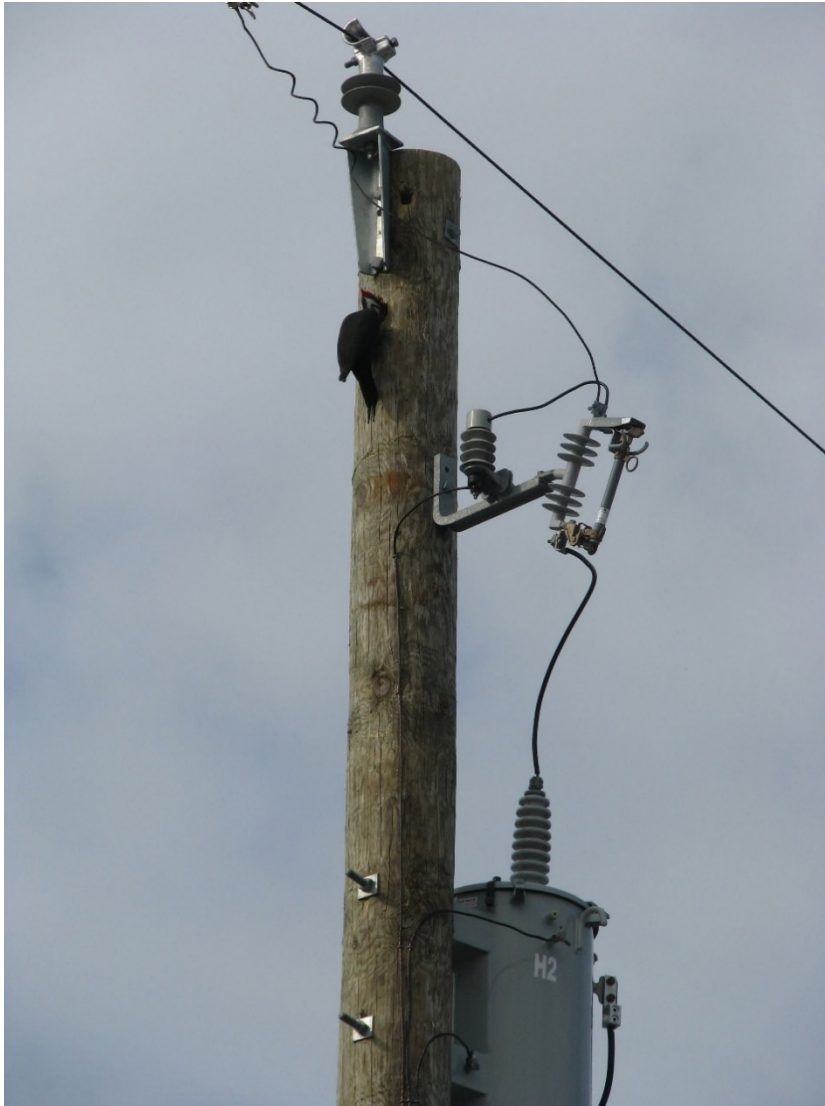
The above photo was taken on March 25th and is a one-month old pole (installed in February 2021) where a woodpecker has already made a hole.
