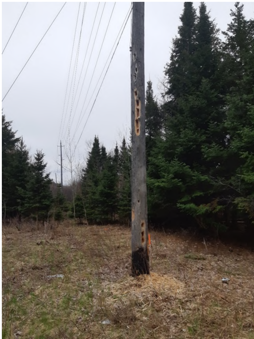
Pole with Multiple Holes in 44kV Sub transmission Line
