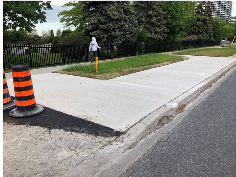
Photo 2: West Side of Bathurst St., South of Kenton Dr. (looking north west). TTC bus stop pad after repair.
