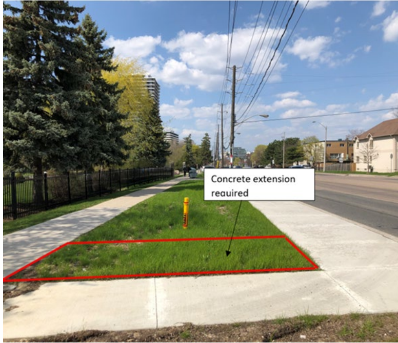
Photo 1: West Side of Bathurst St., South of Kenton Dr. (looking north). TTC bus stop pad prior to repair.
