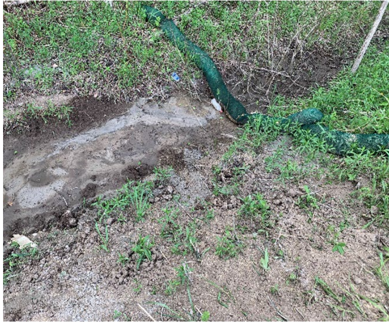
Photo 4a: Silt Soxx™ limiting potential for off-site sedimentation between Flos Road 7 and Flos Road 8 (May 2020).
