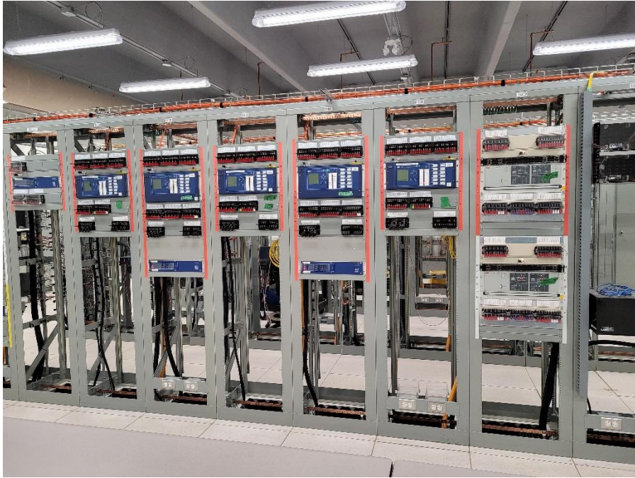
Wawa – new various protection racks
