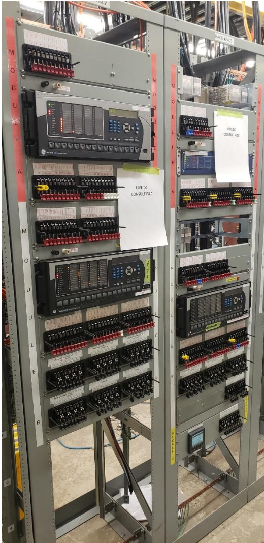
Lakehead - Transformer and Bus A protection rack
