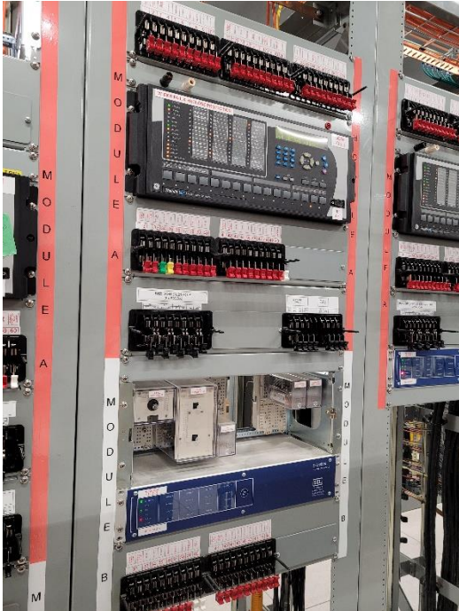
Wawa – new breaker protections
