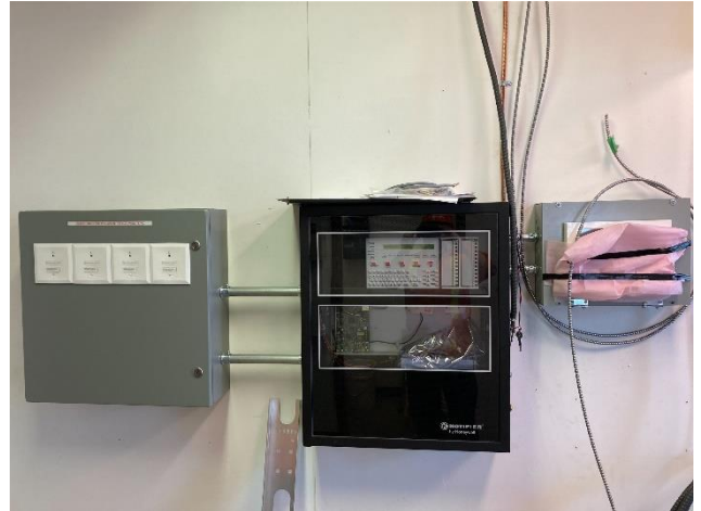
Lakehead TS - newly installed HVAC control panel
