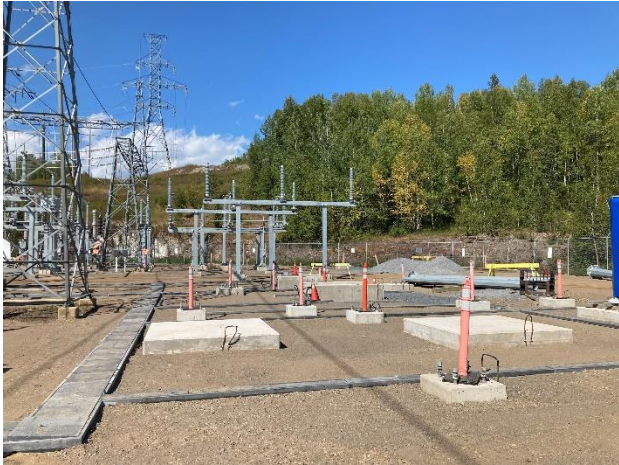
Lakehead TS - newly grounded SC21 area including Cap bank switch, steel and insulators
