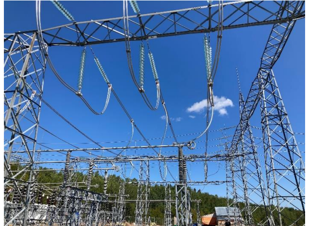
Lakehead TS - newly upgraded strain bus and insulators (P bus and H bus)
