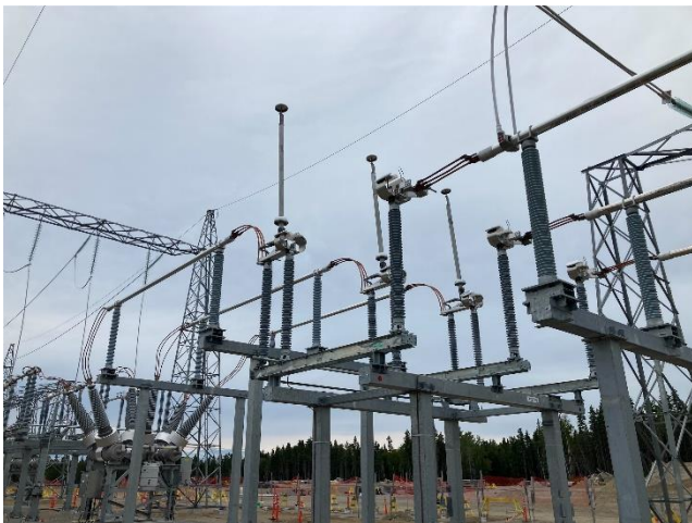
Marathon TS - newly installed strain/rigid bus in Bay 8(East side of yard)
