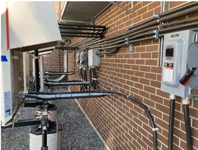
Lakehead TS - Wired HVAC units outside A building
