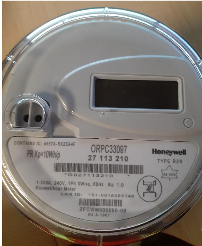
Figure 5-1: Typical ORPC Smart Meter Installation
