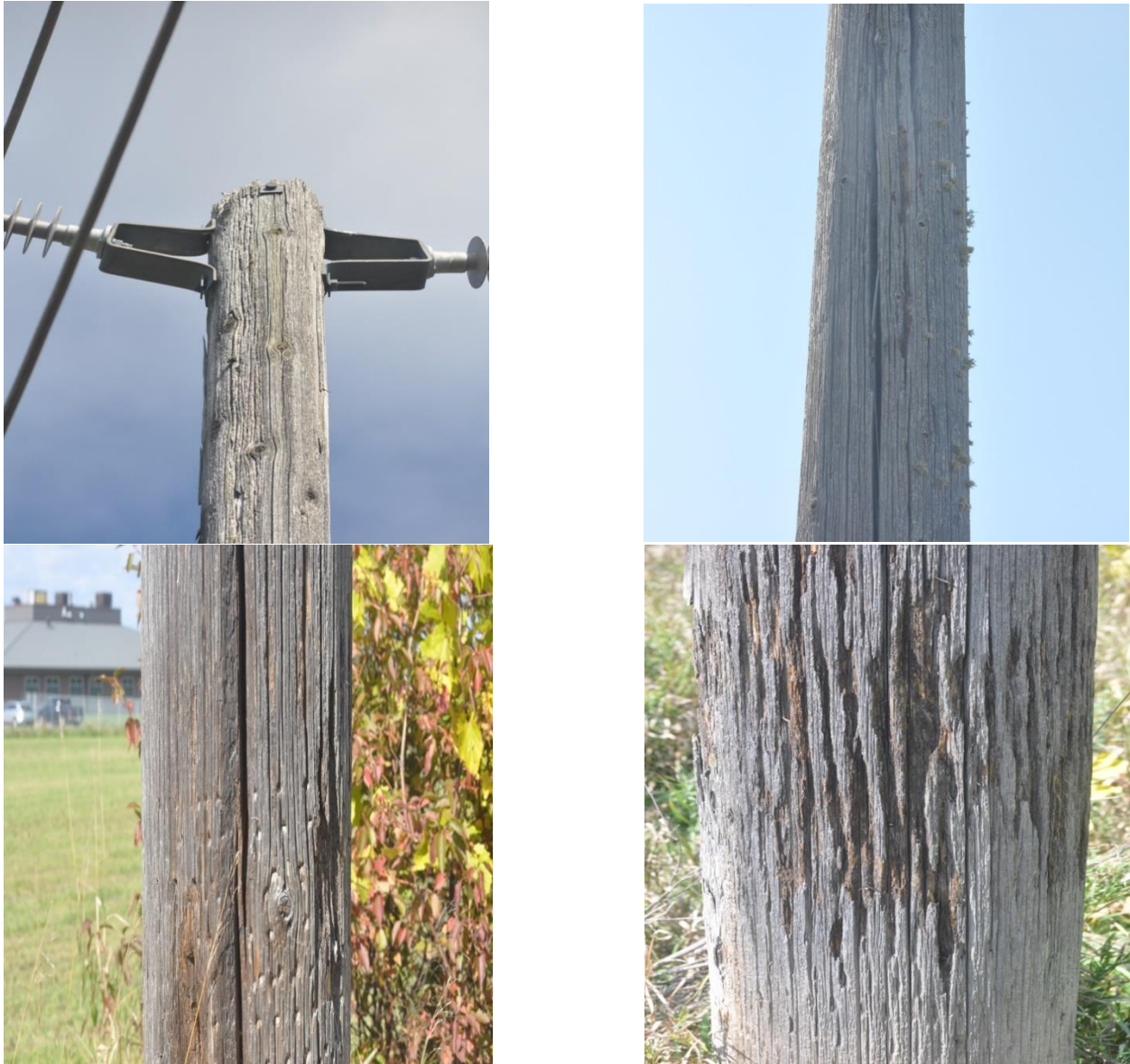
Figure 7-1: Degradation of the 44kV Supply Lines into City of Pembroke
