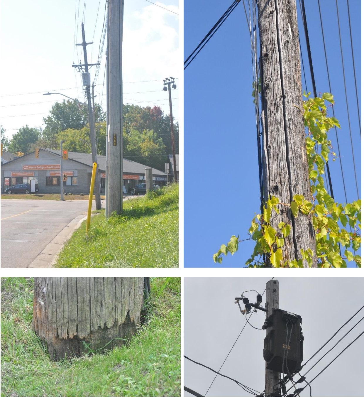
Figure 6-3: Examples of Deteriorated & Aging Overhead Assets
