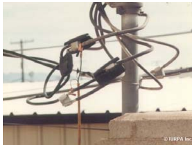
Figure 4-14, Illegal Tap at Service Mast
