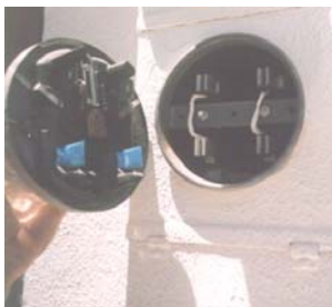
Figure 4-13, Jumpers Installed in Meter Socket
