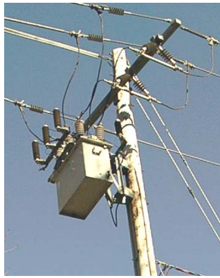
Figure 4-10, Typical Pole-Mounted Automatic Circuit Recloser
