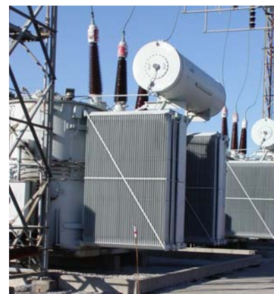
Figure 4-8, Wonderland T.S. Power Transformers
