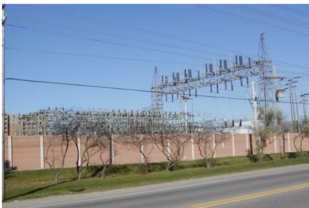
Figure 4-7, Wonderland Transformer Station
