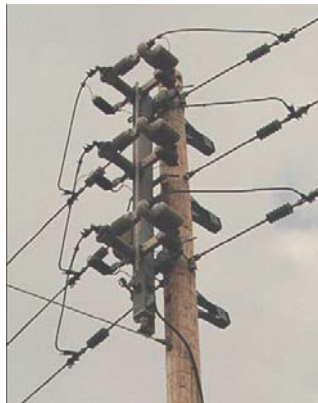
Figure 4-11, Typical Distribution Automation Switch
