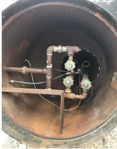
Figure 2: Three burners connected without throttle valves
