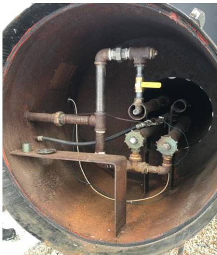
Figure 3: Three burners with throttle valve on 3 rd burner (OFF)
