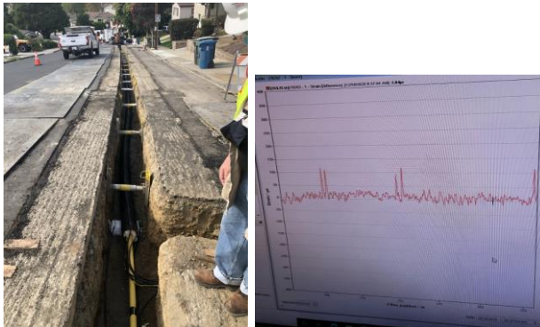
Pilot deployment and Strain Test Signal at a DIMP Fault Crossing Site
