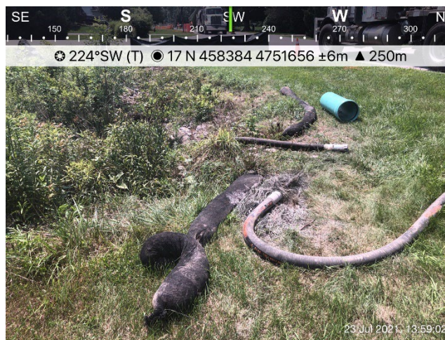
Photo 24: HDD along Falconbridge Drive under WC98. Inadvertent release occurred in cobbly road culvert fill. Silt Soxx™ used to contain spill.
