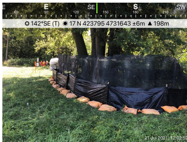
Photo 6: Sydenham River; Silt fencing & turtle exclusion fencing has been installed along upper east bank of river.
