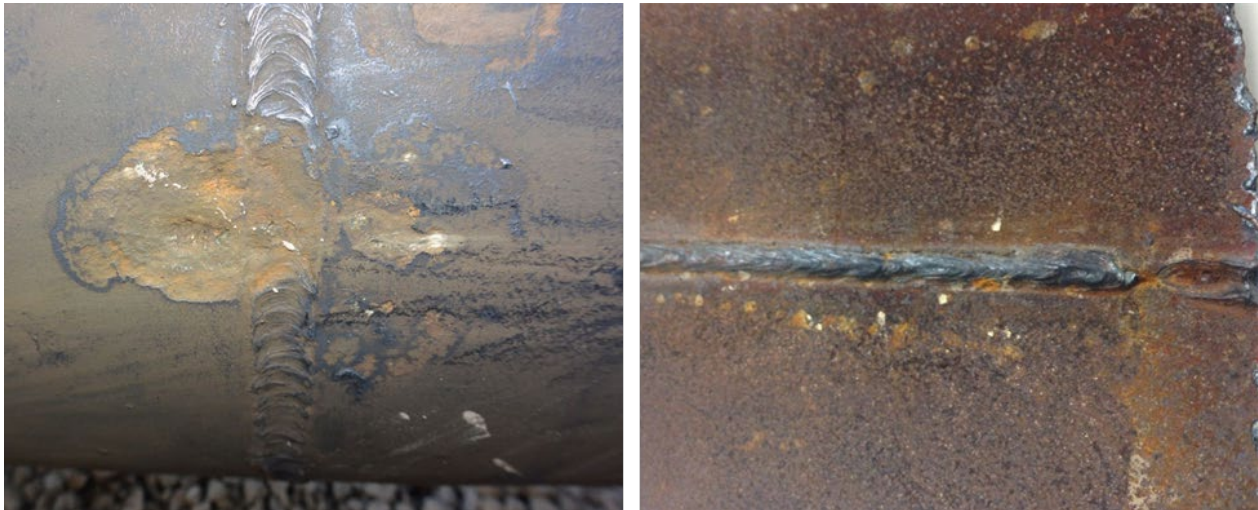
Figure 7: Examples of Failed Installation Welds and Poor Internal Fusion
