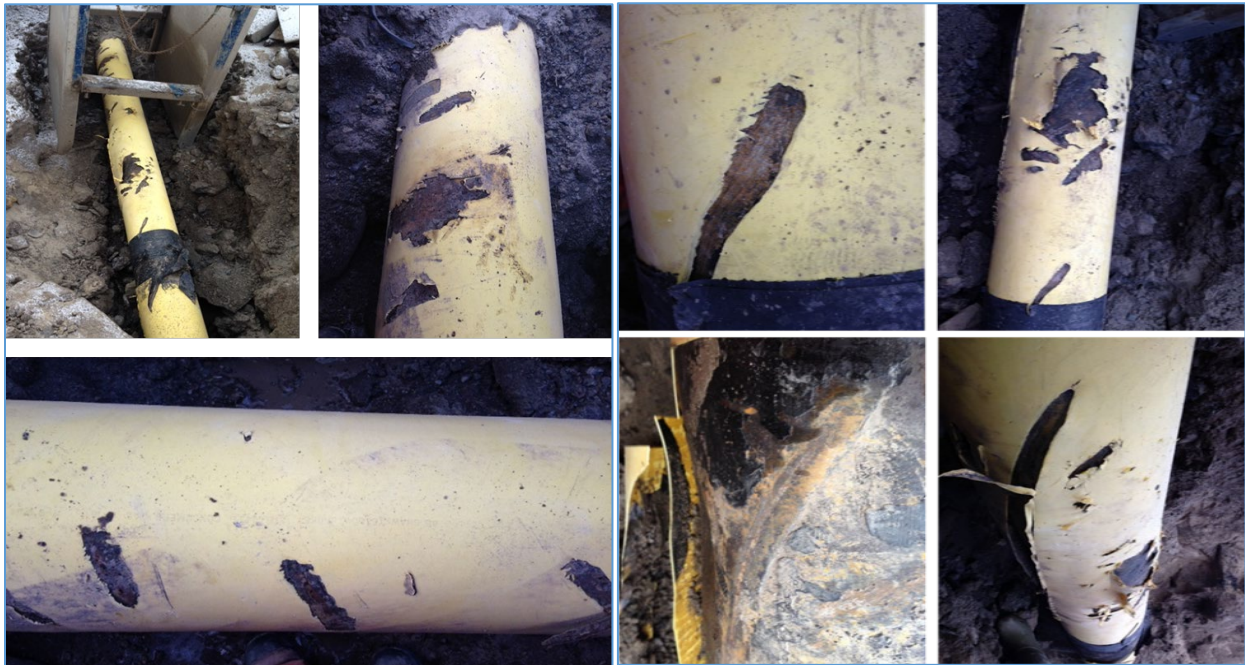
Figure 9: Examples of Damage to the NPS 16 Gas Main
