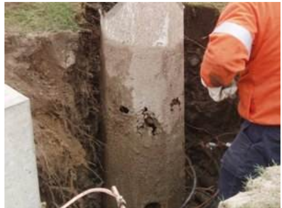
Figure 9 - Sample Corroded Poletran base
