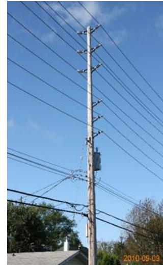
Figure 2: Typical Pole in Project
