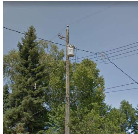
Figure 4: Typical Pole in Project
