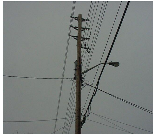
Figure 2: Typical Pole in Project
