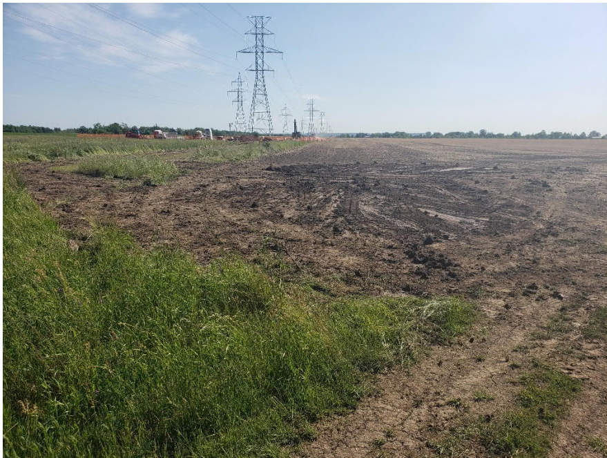
Photo 16: Inadvertent return at KP 21+985 following clean-up, facing southwest.
