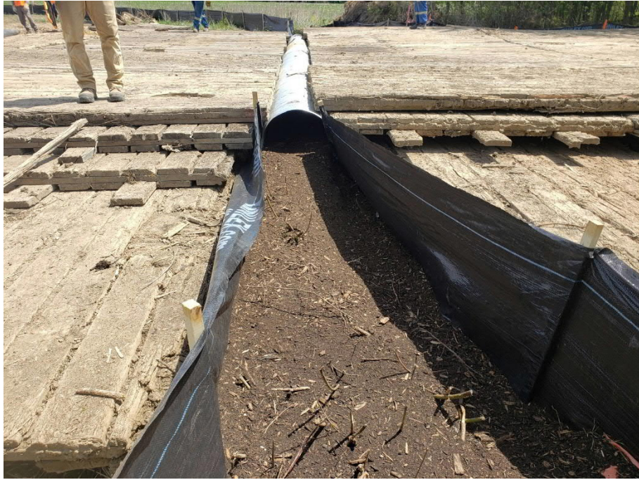
Photo 11: Jefferson Salamander culvert crossing at KP 8+045, view facing north.
