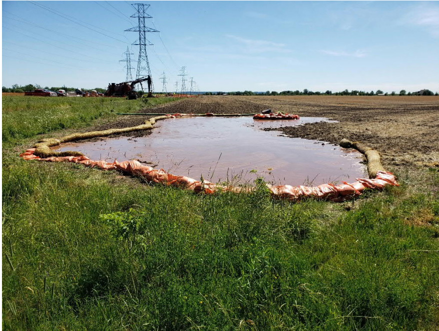
Photo 15: Inadvertent return at KP 21+985 contained using sediment control measures, facing southwest.
