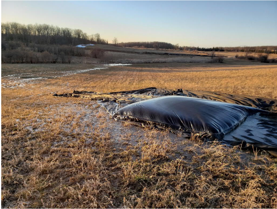
Photo 5: Silt bag used during dewatering at KP 8+630 to prevent erosion and sedimentation, view facing northwest.
