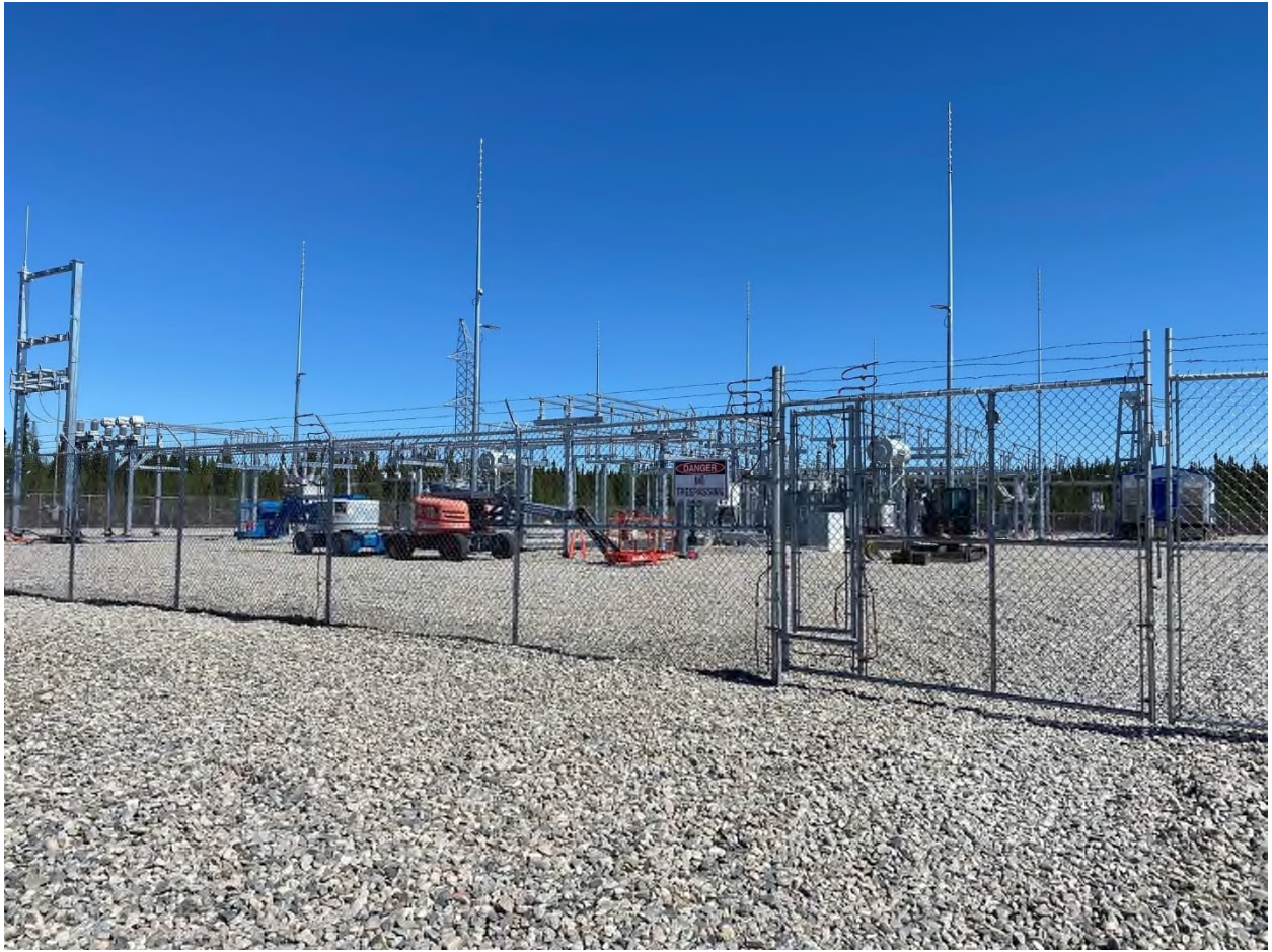
Photo 8: Substation D – North Caribou
