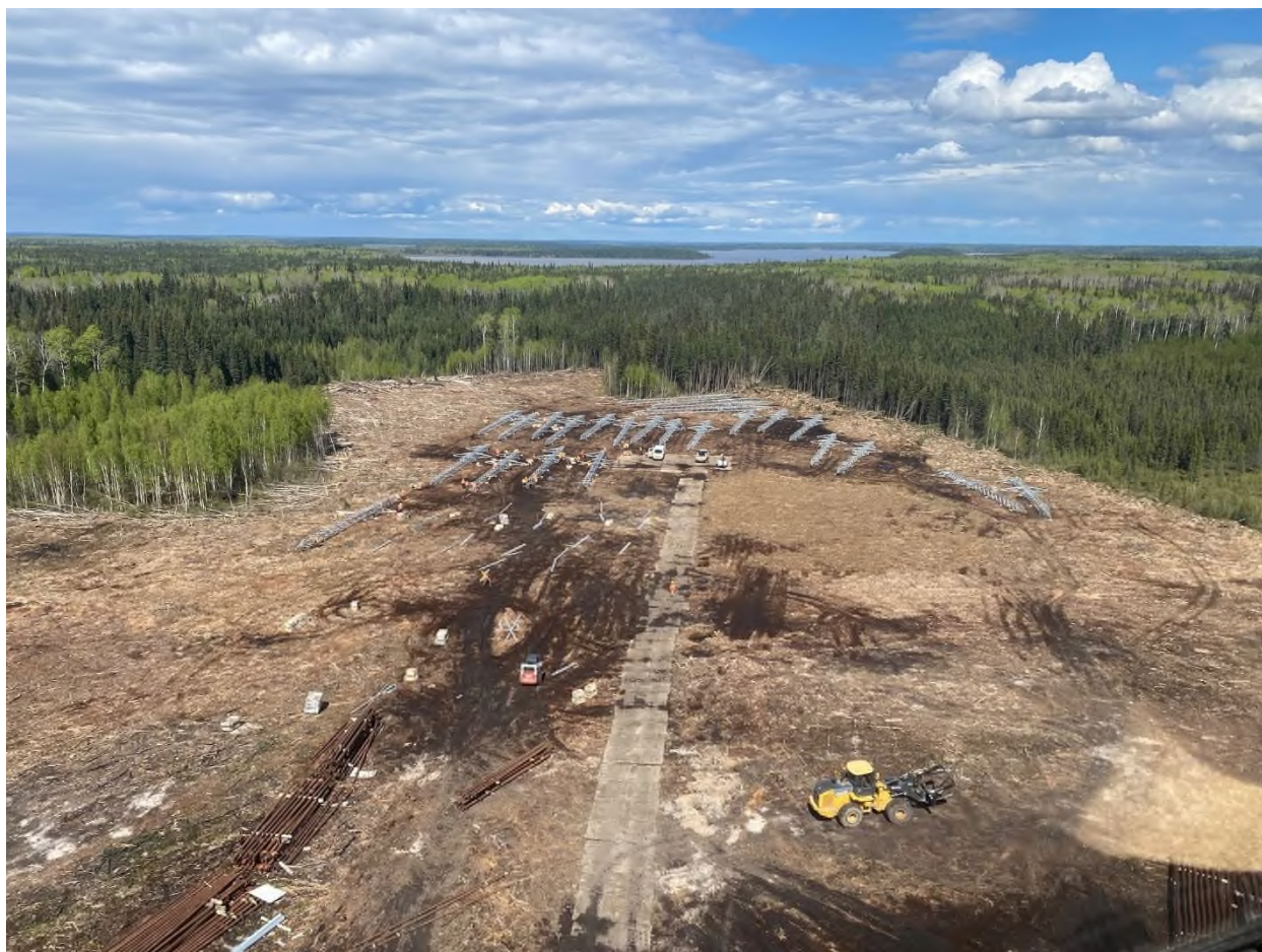
Photo 3: Substation Z – Sandy Lake yard
