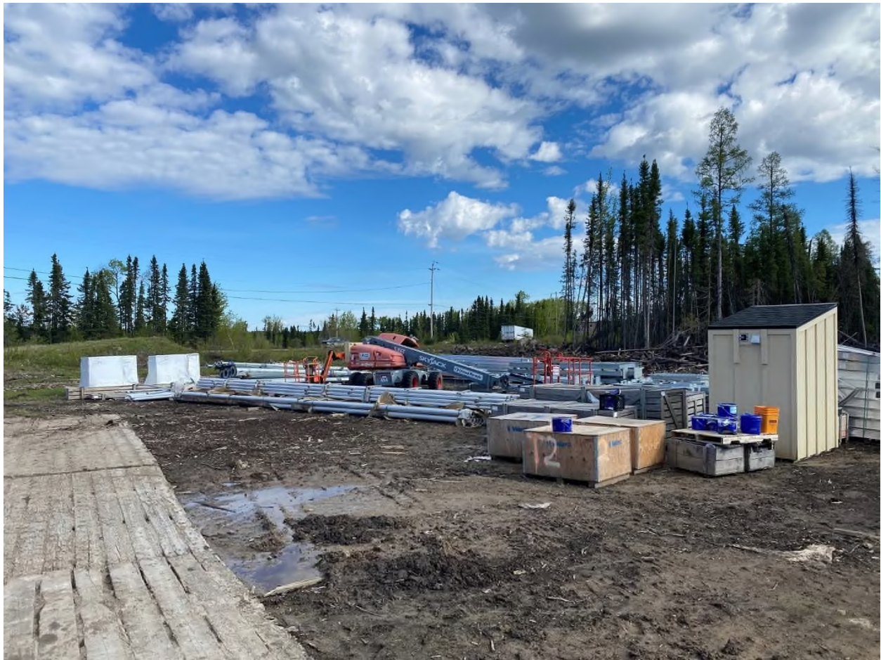
Photo 9: Substation U – Deer Lake
