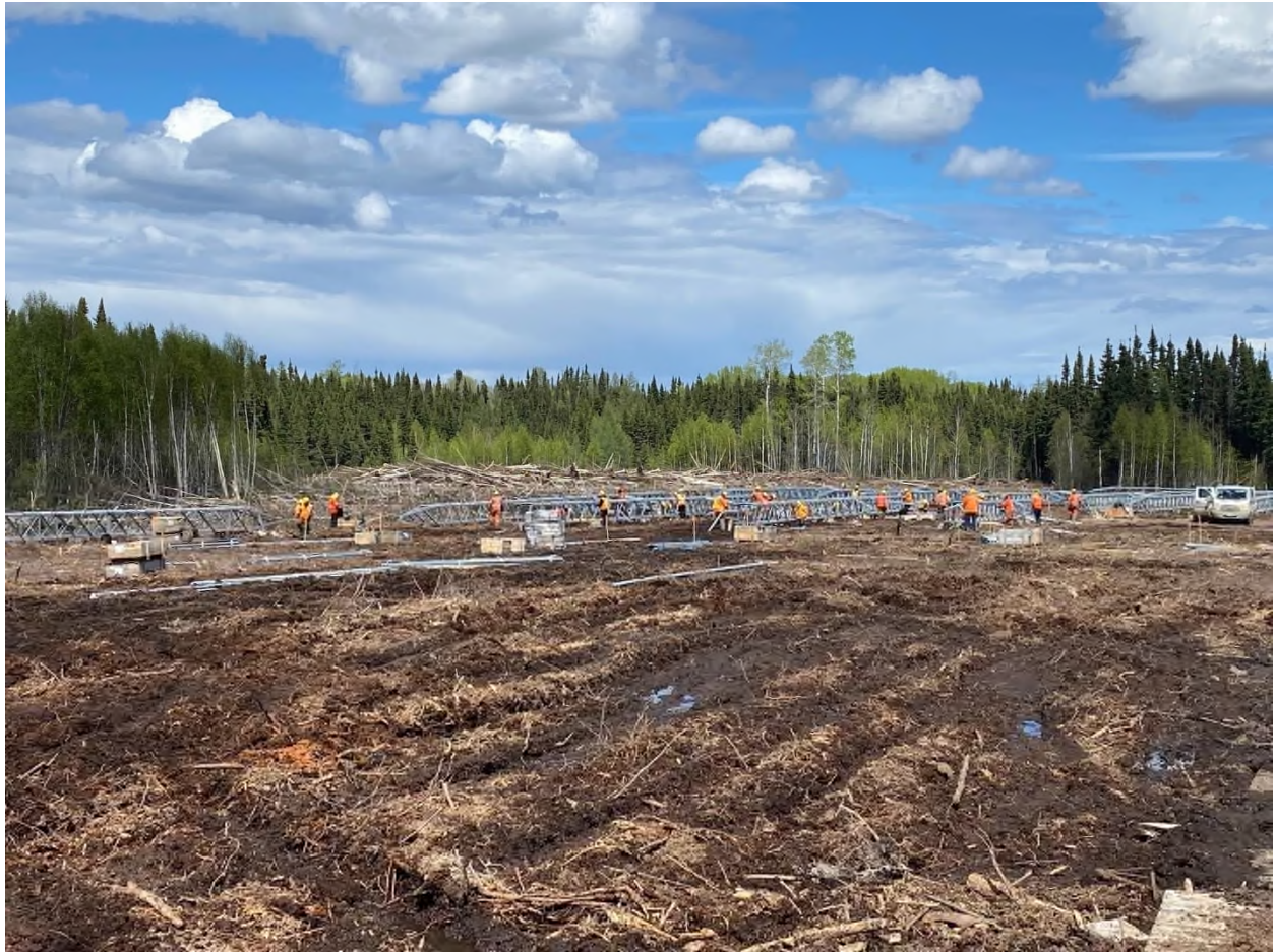
Photo 7: Substation Z – Sandy Lake assembly
