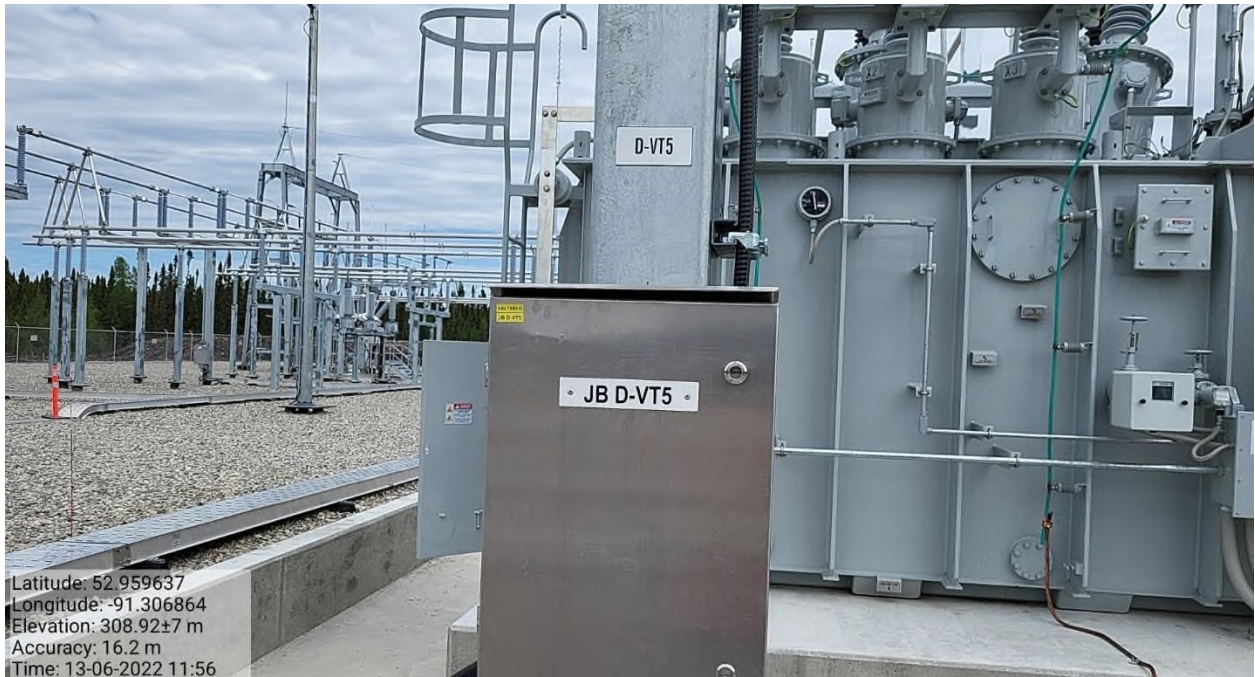
Photo 17: Substation D – ID affixation
