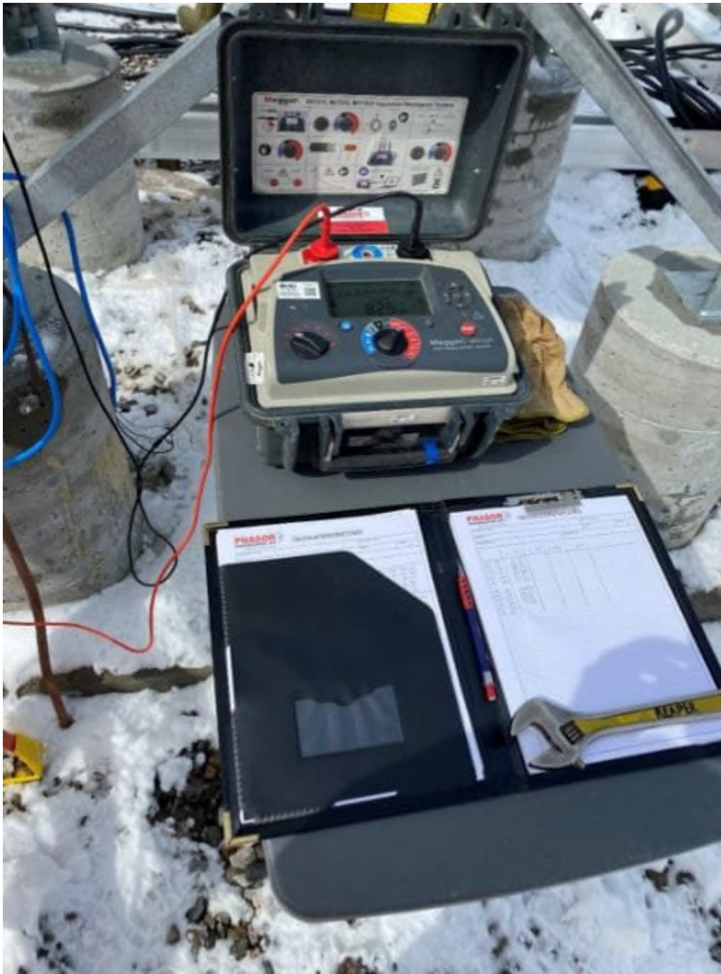
Photo 11: Breaker testing at Sub J Kingfisher
