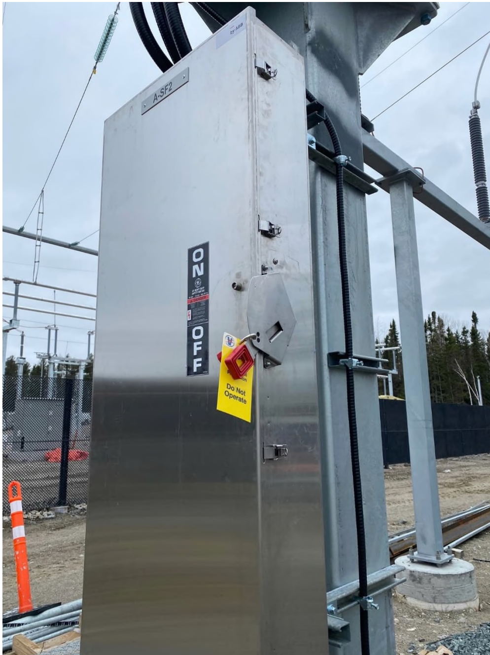
Photo 5: Substation A SSVT panel locked and tagged
