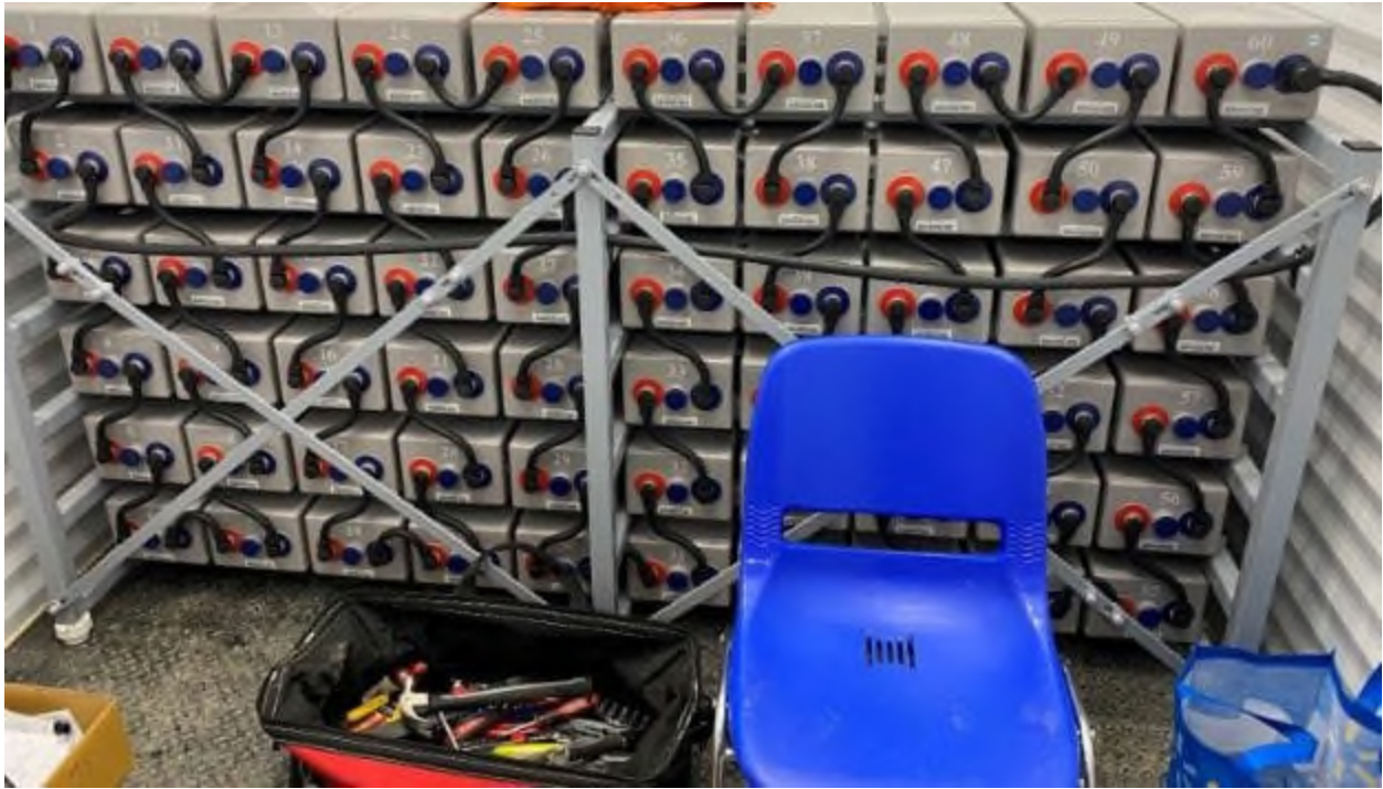
Photo 6: Batteries installed at Sub A
