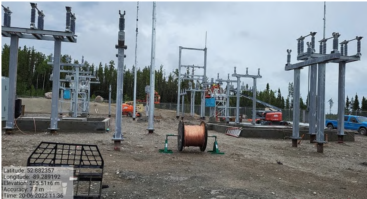
Photo 18: Substation I – Wunnumin Steel structures and insulators
