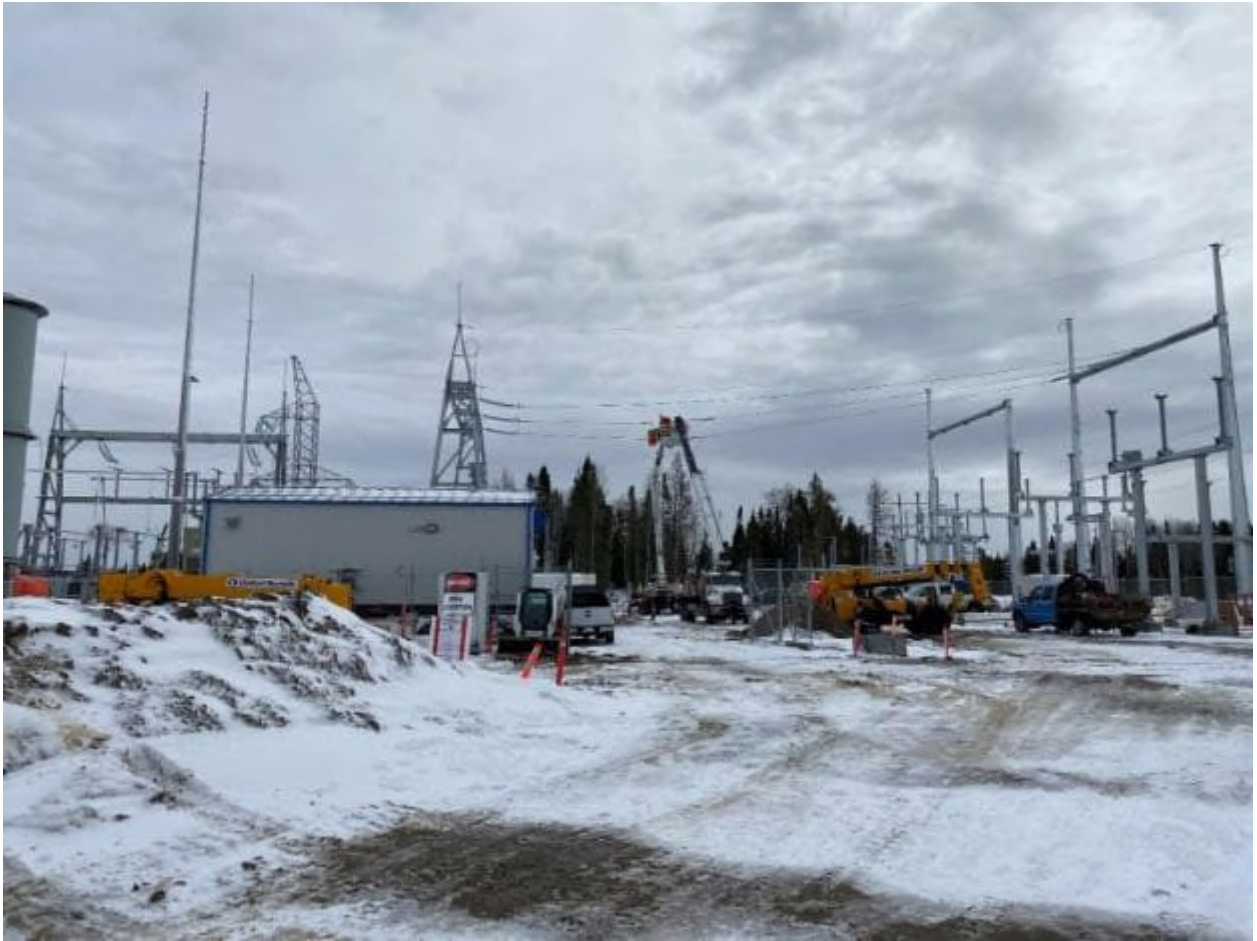
Photo 5: A-frame 3L3 span from Sub A to HONI Sub
