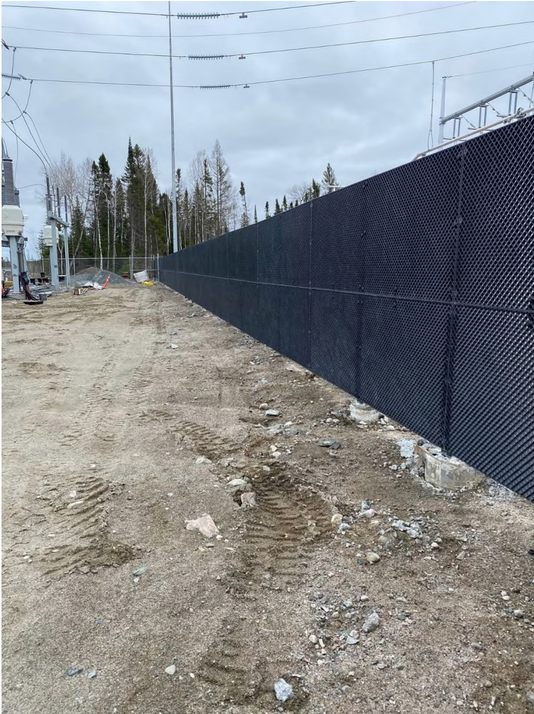
Photo 3: Substation A insulative fence
