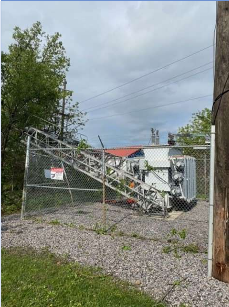
1 Figure 5: Uxbridge TS 2 Location; Brock St West 3 Date: May 22, 2022 4 5 Municipal Substation damaged by strong winds 6 7 8 9
