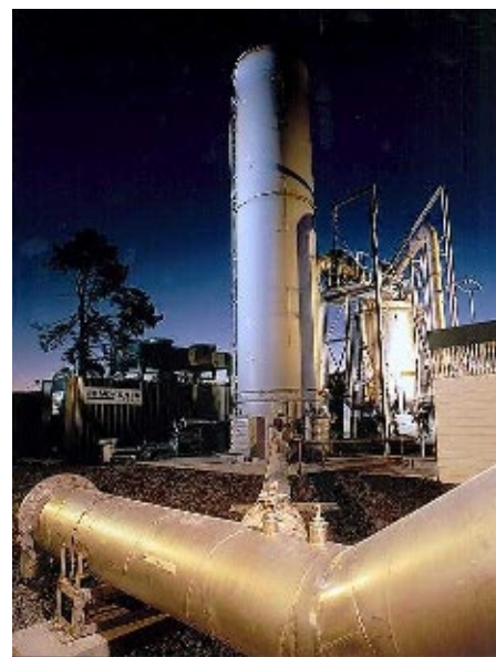
Figure 3-10. Submerged Combustion Leachate Evaporator
