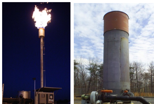
Figure 1-4. Open (left) and Enclosed (right) Flares
