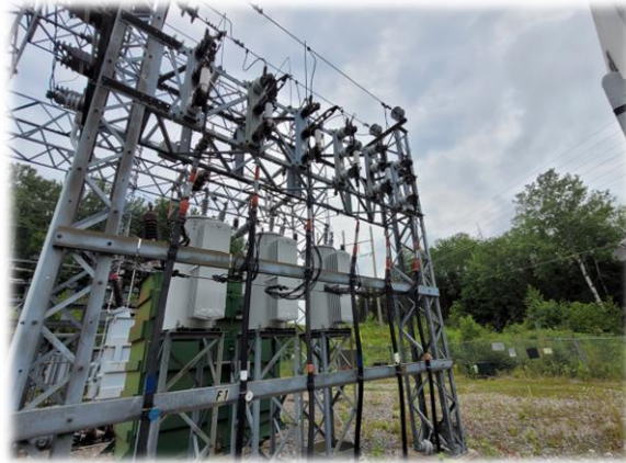
Fuses on Station Structure
