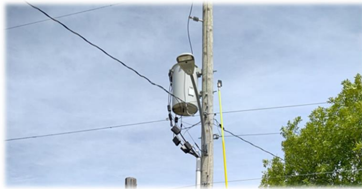
A Pole-Mounted Transformer
