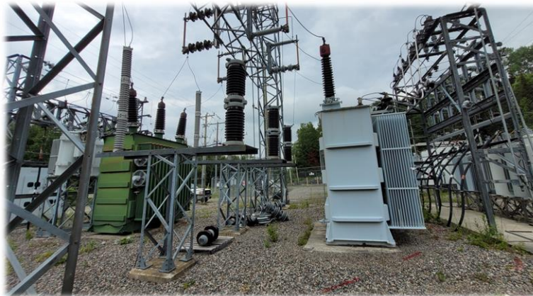
Side View of Both Transformers
