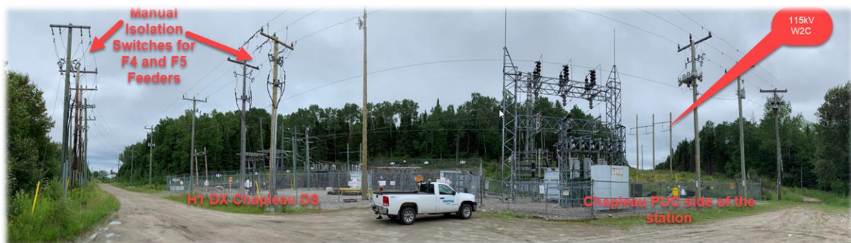
Panorama View of Hydro One & Chapleau Stations
