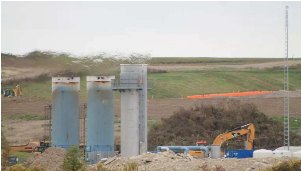
Methane gas can be seen coming from the stacks over an organic waste pile at the Ridge Landfill near the town of Blenheim, Ont. (Amy Dodge/CBC News)
