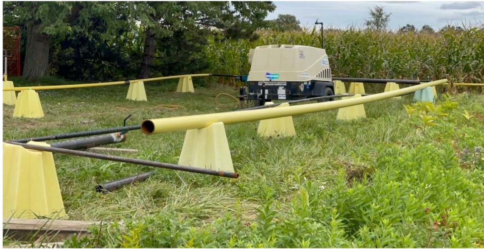
Parts of the pipeline under construction that will be used to convert methane gas from organic waste into renewable natural gas. (Amy Dodge/CBC News)
