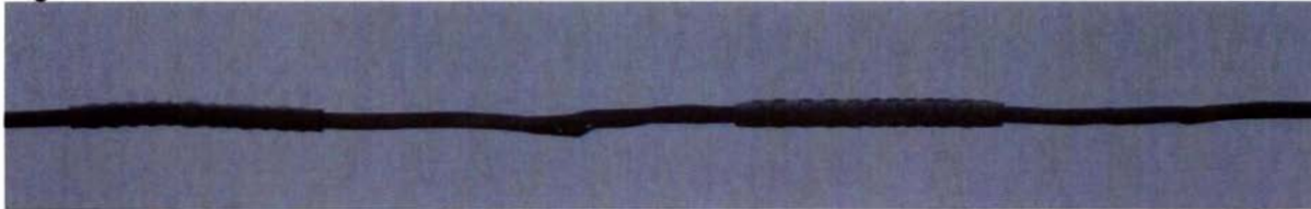
Figure 16 Conductor in Poor Condition
