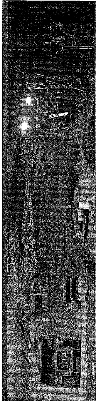
Musselwhite Mine Electrical Power Supply
