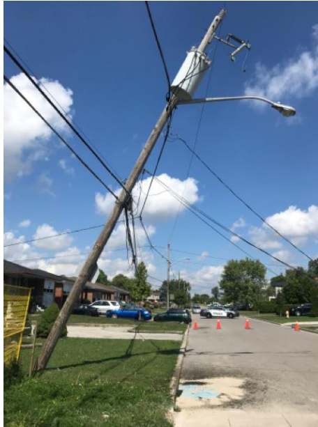
Figure 6: shows a leaning distribution pole Grid Response crews attended to and forwarded for permanent reactive repair (2021)
