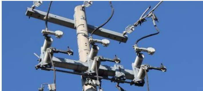
5 Figure 8: Manual Gang-Operated Switch
