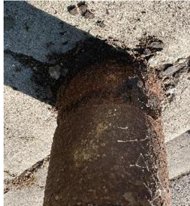
4 Figure 5: Corrosion on Steel Pole Base
