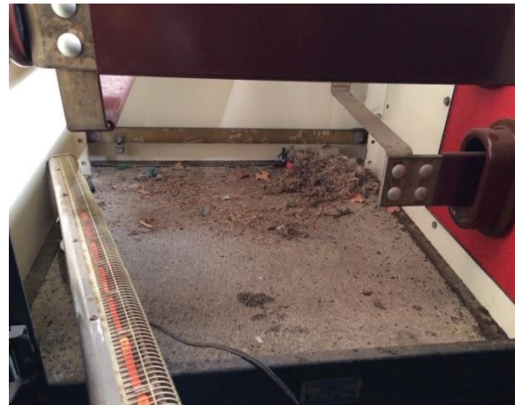
Figure 16: Pests Inside Outdoor Switchgear
