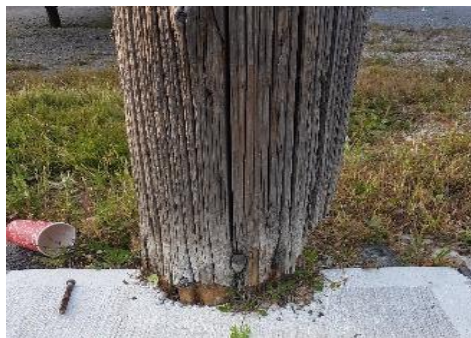
10 Figure 3: Rot at Base of a Pole
