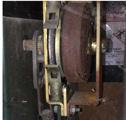
Figure 15: Padmounted Switch with Rusted Coil Spring
