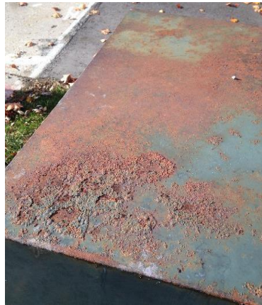
Figure 14: Padmounted Transformer with Surface Corrosion
