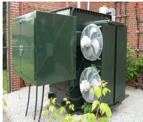
Figure 20: Power Transformer at Neilson Dr. MS
