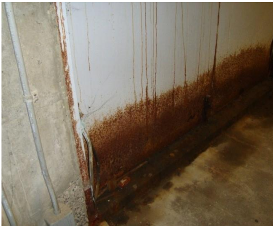
Figure 15: Rusty Switchgear Enclosure
