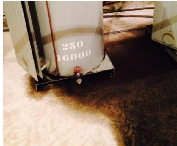
Figure 3: Transformer Leaking Oil
