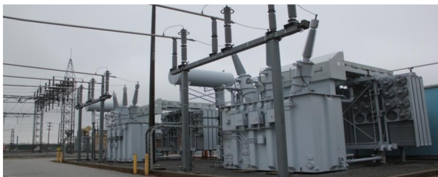
Figure 8: The Station Yard at Cavanagh TS
