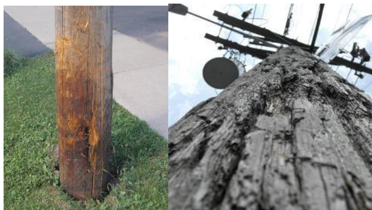
11 Figure 4: (Left) Cracked Wood Pole, (Right) Surface Rot on Pole
