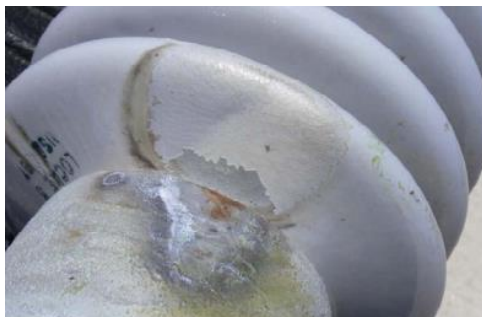
19 Figure 12: Close-up of Damaged Porcelain Insulator Showing Tracking
