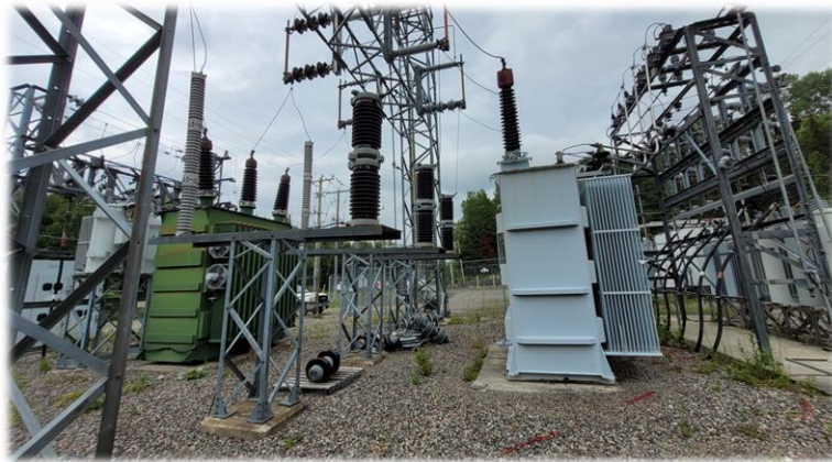
Side View of Both Transformers
