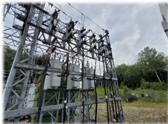
Fuses on Station Structure
