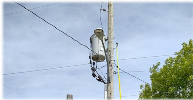
A Pole-Mounted Transformer
