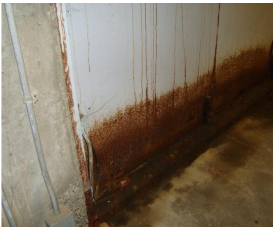
Figure 15: Rusty Switchgear Enclosure
