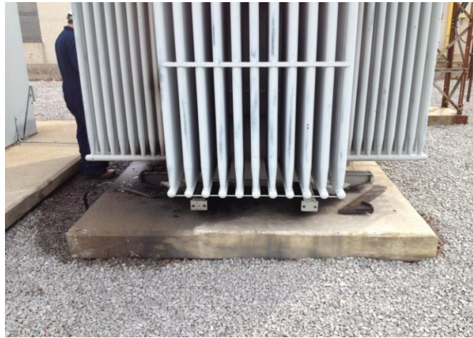
Figure 11: Oil Leak on a Station Transformer
