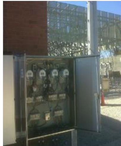
Figure 18: Wholesale Meter Installation at Transformer Station.
