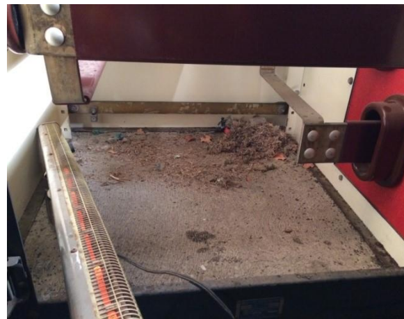
Figure 16: Pests Inside Outdoor Switchgear
