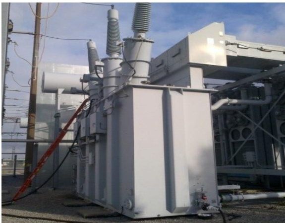
Figure 19: Power Transformer at Cavanagh TS
