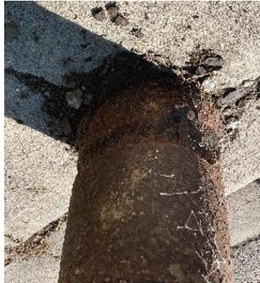
4 Figure 5: Corrosion on Steel Pole Base
