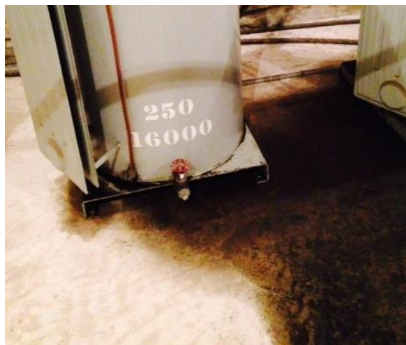
Figure 3: Transformer Leaking Oil
