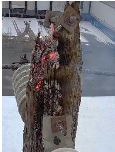
10 Figure 13: Pole fire on December 22nd, 2017
