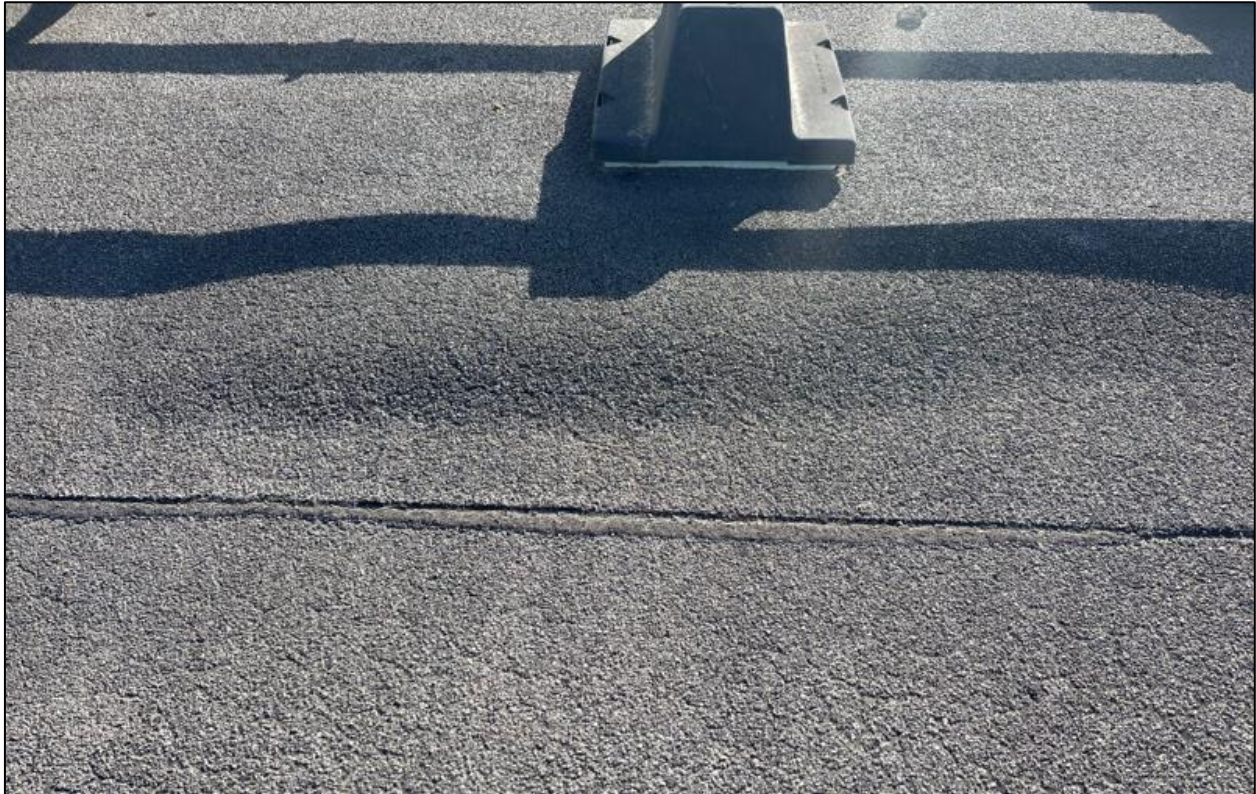
Blisters forming in roofing membrane
