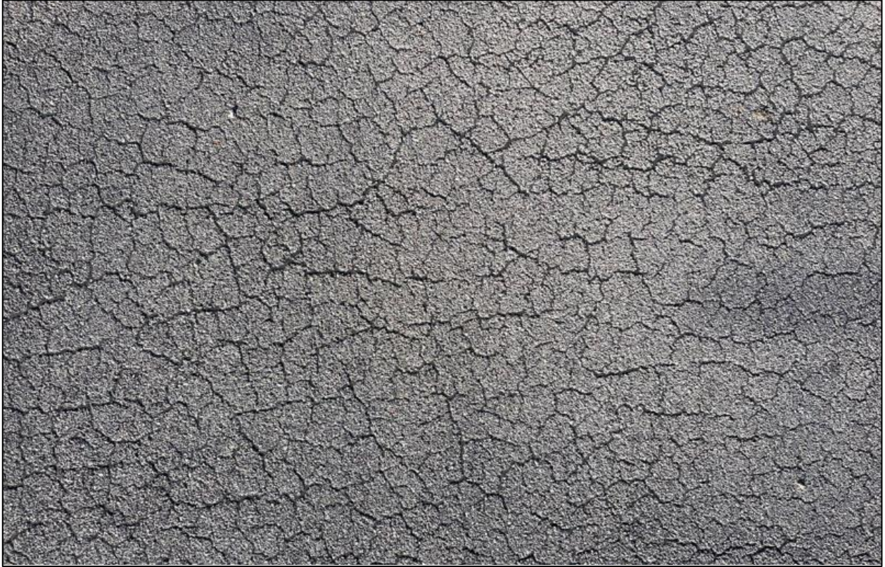
Membrane is cracking and alligatoring due to age and weathering
