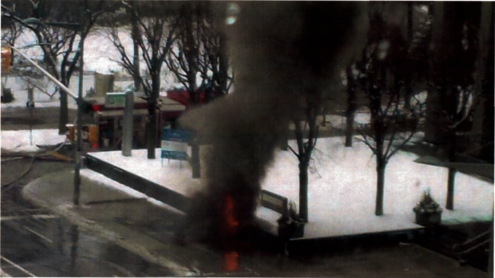
Fibertop Network Protector Vault Fire, January 28, 2013 Vault Location 4651 – 95 St. Clair Ave W.
