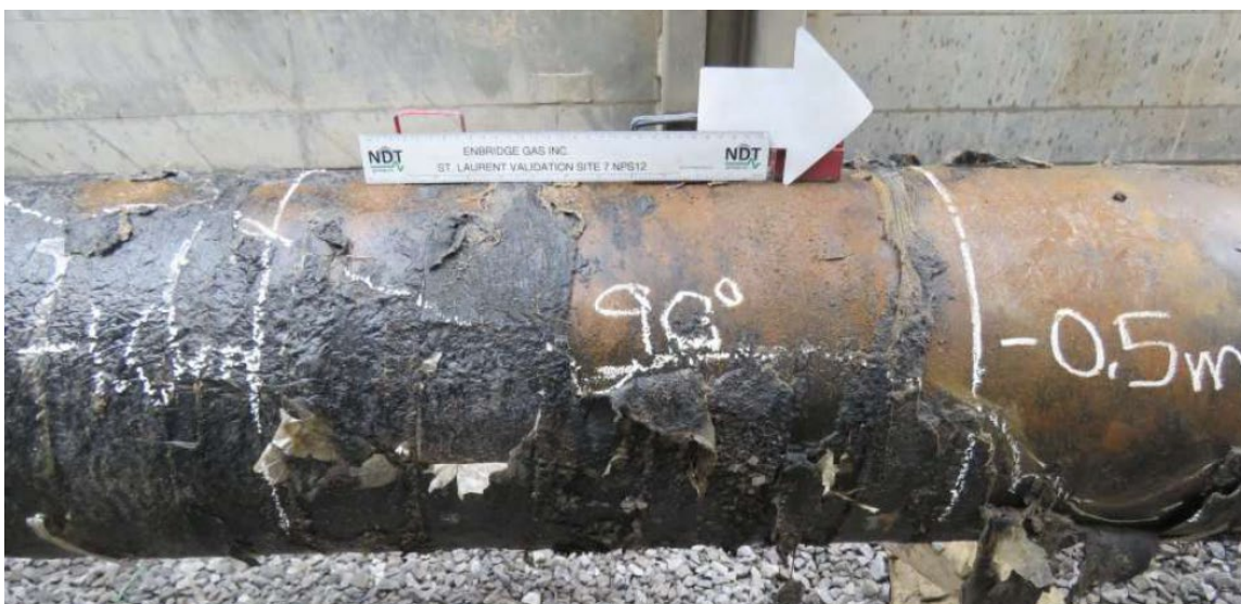
Figure 5: Dig Site 7 - Coating Damage
