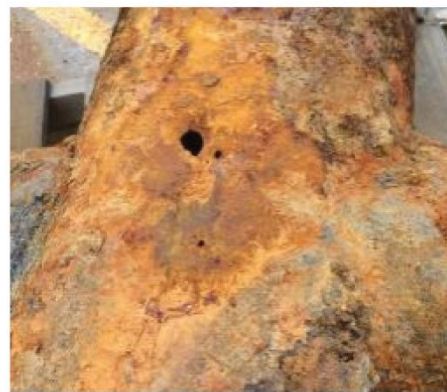
Steel pipeline with corrosion failure
