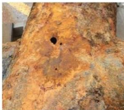
Steel pipeline with corrosion failure
