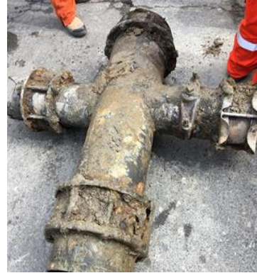
Figure 6.2-19: Detail of fabricated fitting after removal
