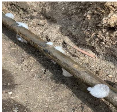
Figure 6.2-39: Leaking bare and unprotected pipe (soap bubbles indicate leak points)
