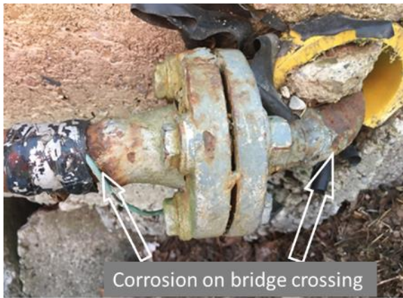
Figure 6.2-8: Severe corrosion on bridge-crossing pipe
