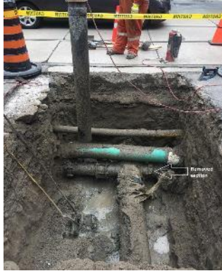
Figure 6.2-18: Leak investigation on vintage NPS 12 gas main
