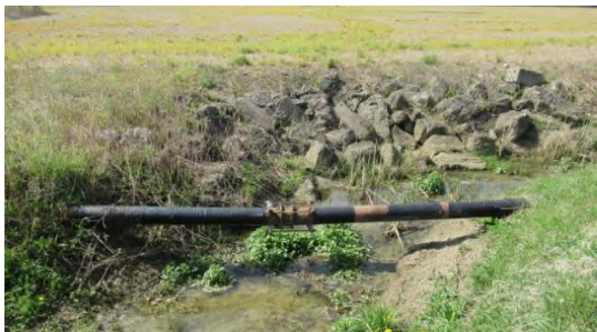
Figure 6.2-12: Aerial crossing with exposed mechanical fitting
