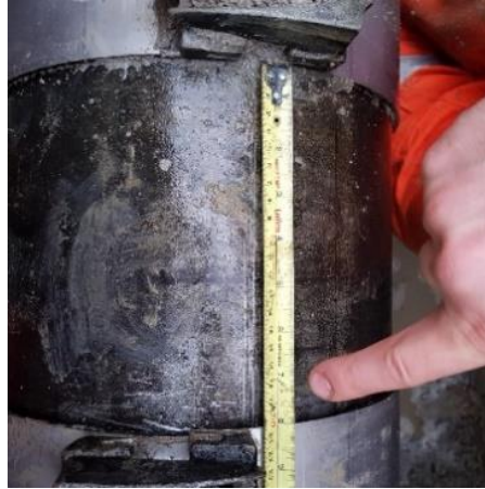
Figure 6.2-45: Corrosion Pitting from TTC Stray Current
