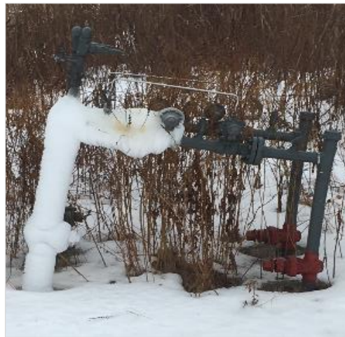
Figure 6.2-55: The Joule-Thomson Effect on a District Station
