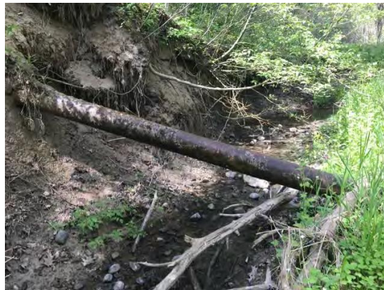
Figure 6.2-14: Erosion increasing the unsupported length of an aerial crossing
