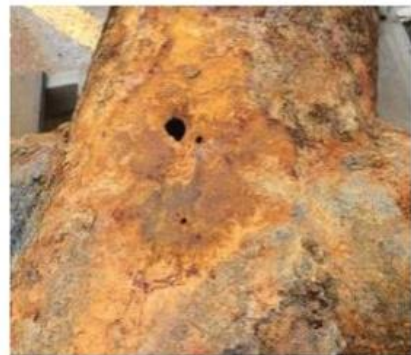
Steel pipeline with corrosion failure
