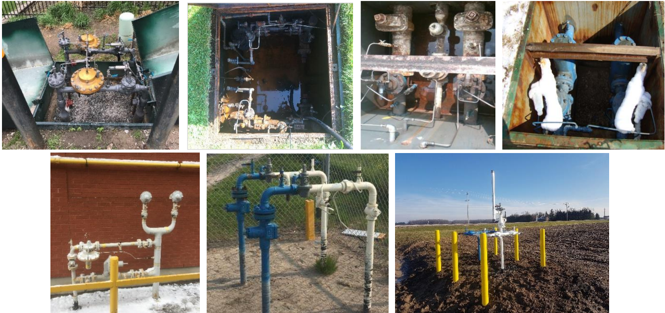
Figure 6.2-51: Examples of Distribution System Stations
