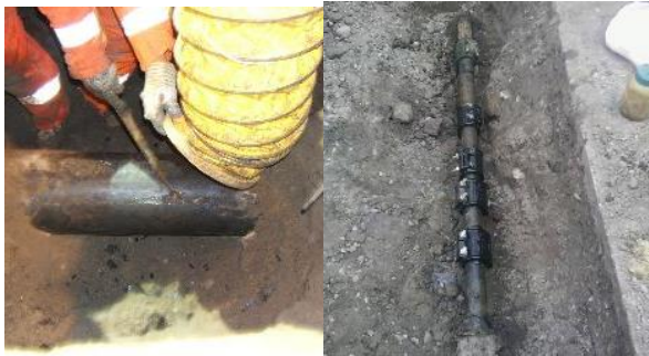
Figure 6.2-6: Bare and unprotected steel failures
