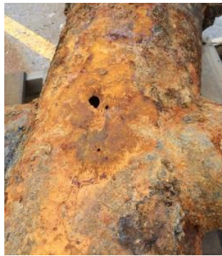
Figure 6.2-20: Multiple leaks due to severe corrosion on vintage NPS 12 gas main
