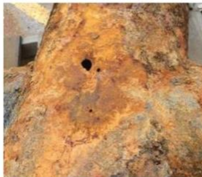
Steel pipeline with corrosion failure
