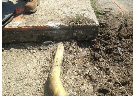
Figure 6.2-7: Shallow and embedded gas main due to road grade change
