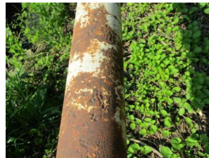
Figure 6.2-13: Coating degradation and corrosion pitting
