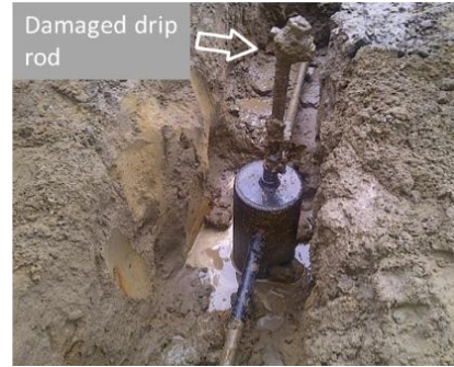
Figure 6.2-11: Damaged drip rod on vintage NPS 2 gas main
