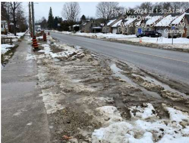
Photo 35 Additional restoration will be required in Spring of 2025
