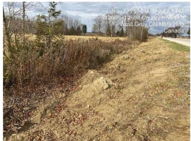
Photo 16 Rough grading has been completed prior to potential settling. Additional restorative measures will be required in spring 2025.
