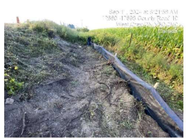
Photo 6 Silt fence in use to isolate disturbed ROW after backfilling of trench.
