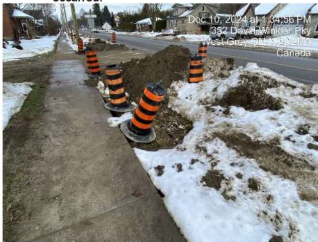
Photo 27 Settling occurred along boulevard where open cut installation work was completed.
