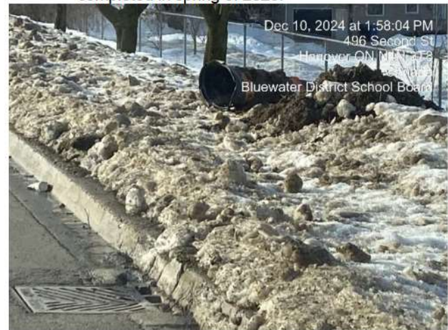
Photo 30 Residual stockpile of backfill remaining on boulevard. Restorative measures to be completed in 2025
