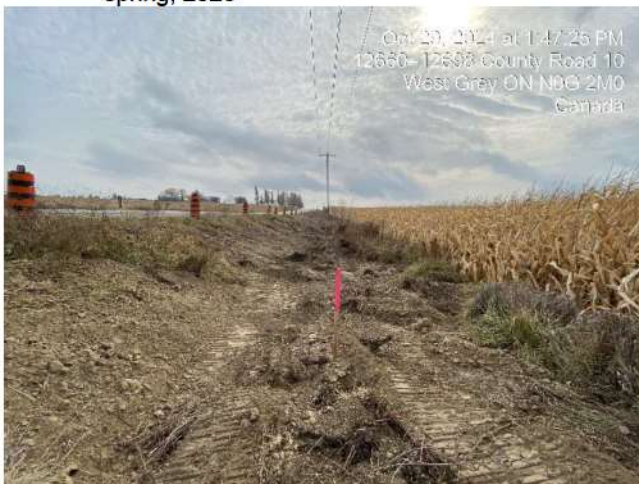
Photo 15 Rough grading after backfilling of trench. Additional grading potentially will be required after settling in spring 2025.
