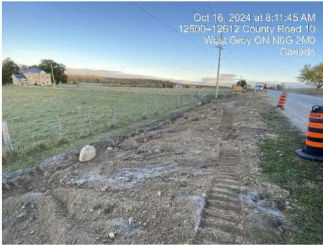
Photo 13 Rough grading completed prior to settling. Additional restorative measures will be required in spring, 2025
