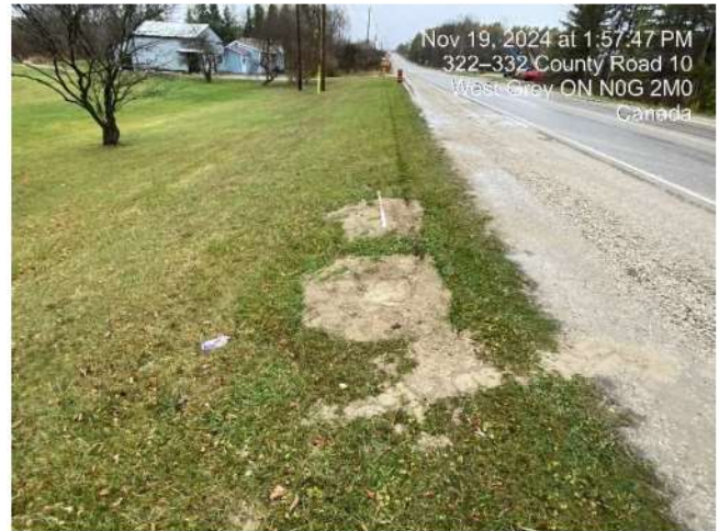
Photo 22 Backfilling of relief pits completed with sand. Settling will require monitoring in spring 2025.
