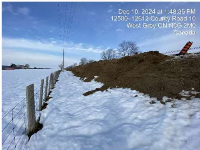
Photo 29 Backfilling of open cut section completed. Restorative measures to be completed in spring 2025.
