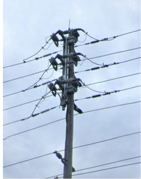
Figure 20: Existing ScadaMate Installation
