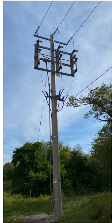
Figure 5: BHI Concrete Pole
