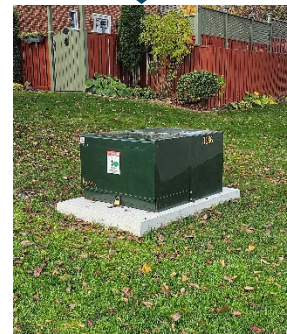
Figure 21: Transformer T186 Pilot Conversion
