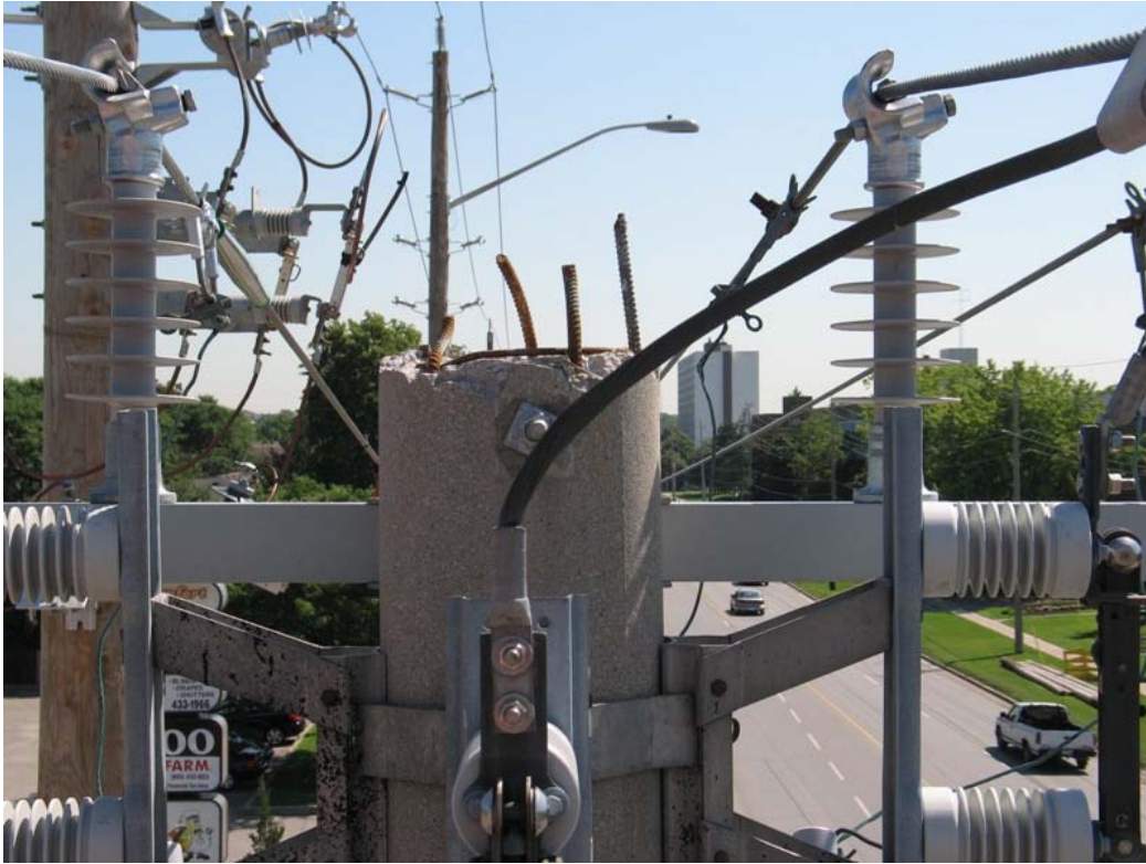
Figure 5: Existing portion of the broken pole
