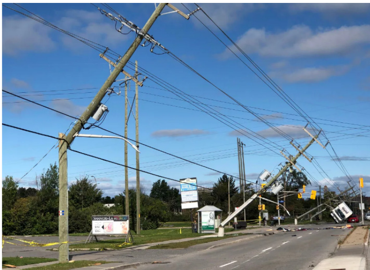
Several poles collapsed along Greenbank Road and Hunt Club Road after a tornado hit Ottawa on Sept. 22, 2018. (Leah Hansen/CBC)
