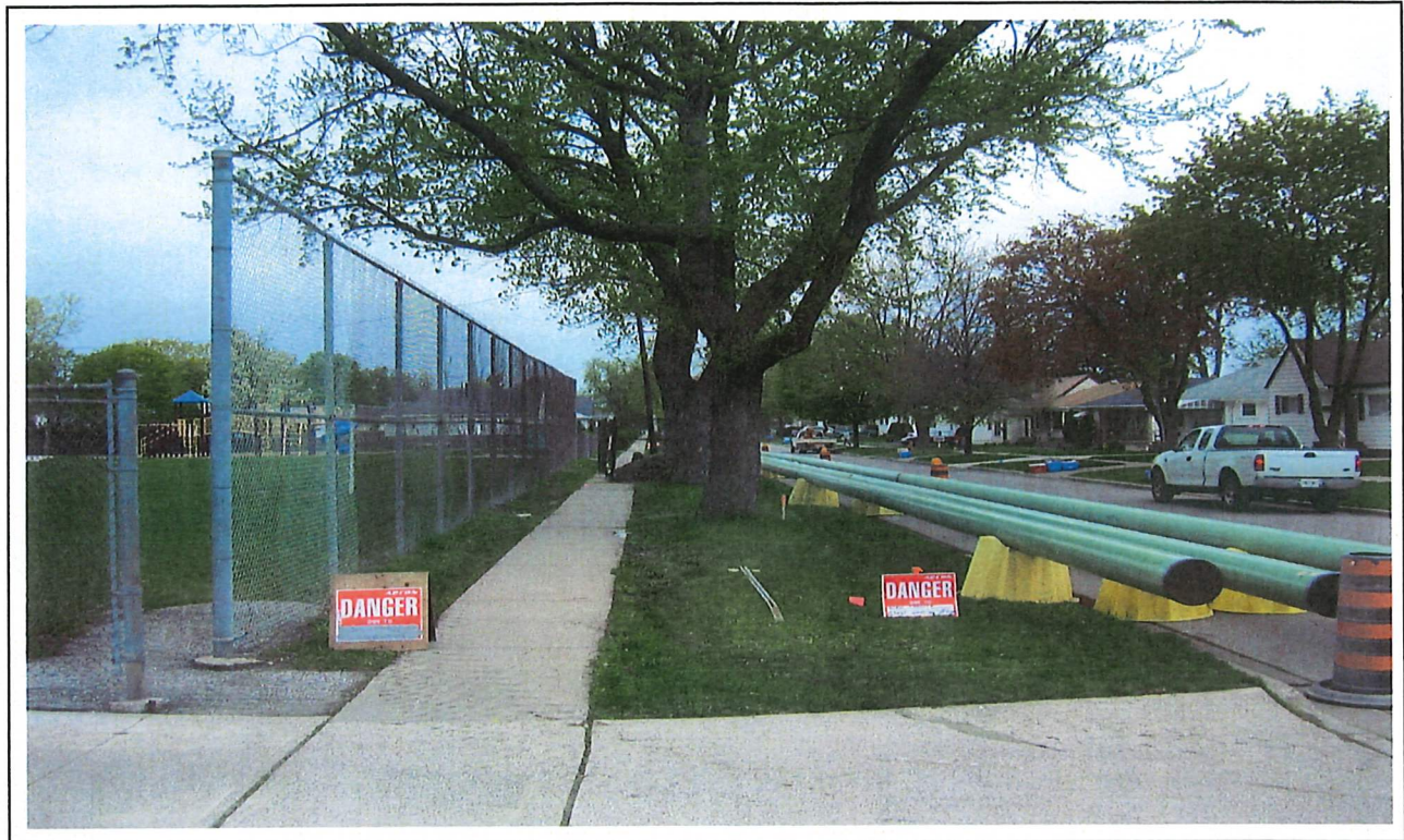
Signs were posted whenever sidewalks were obstructed to inform pedestrians of possible hazards.
