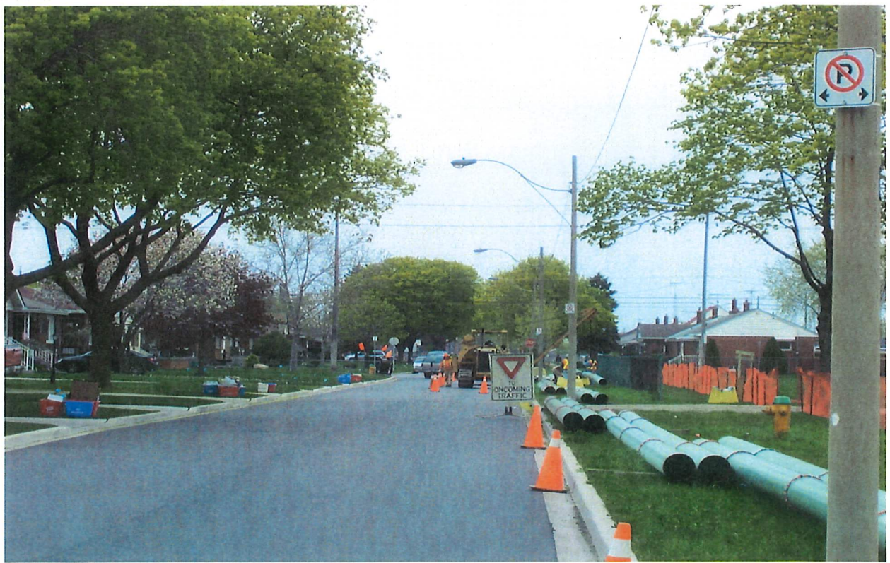
During construction on city streets, one lane of traffic was maintained where ever possible.
