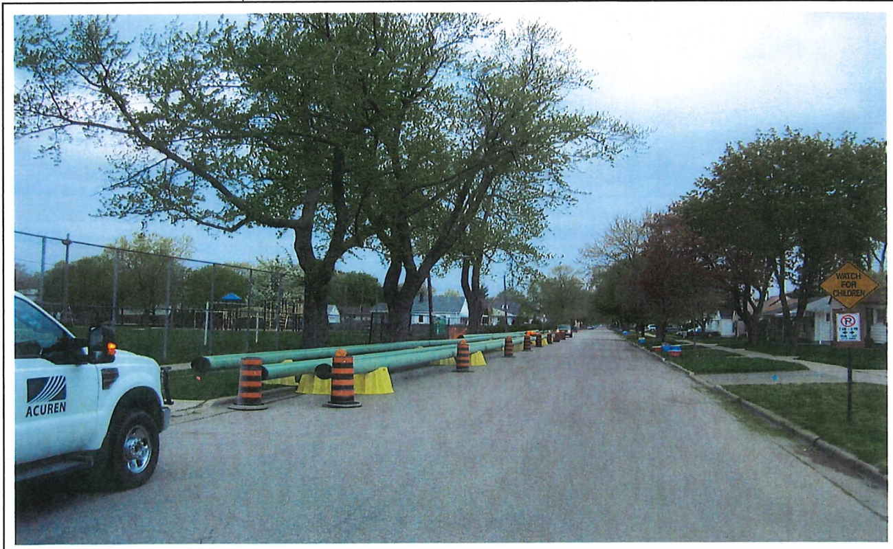
Whenever possible, pipe was stored in front of non-residential areas to allow access to driveways. In this case, the pipe was strung and welded in front of city parkland.
