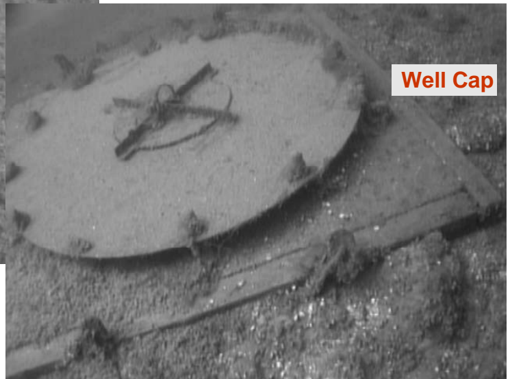
Figure 3.21 - Video still frame images of the intake pipes located east of Sand Bay. The well cap is located at the end of the western most intake pipe as shown in the top image.
