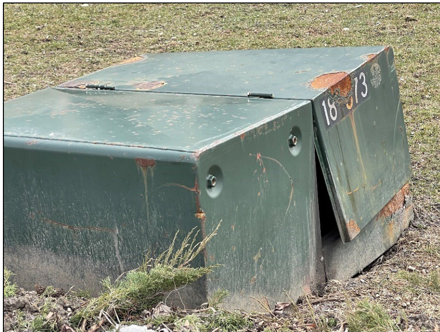
Figure 5.3.3 - 5 Compromised Transformer Enclosure Posing Public Safety Risk
