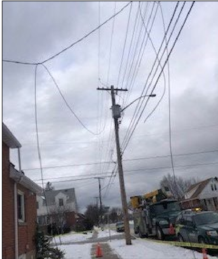
5 6 Figure 5.3.2 - 43 Hamilton – Fallen Undersized Wire
