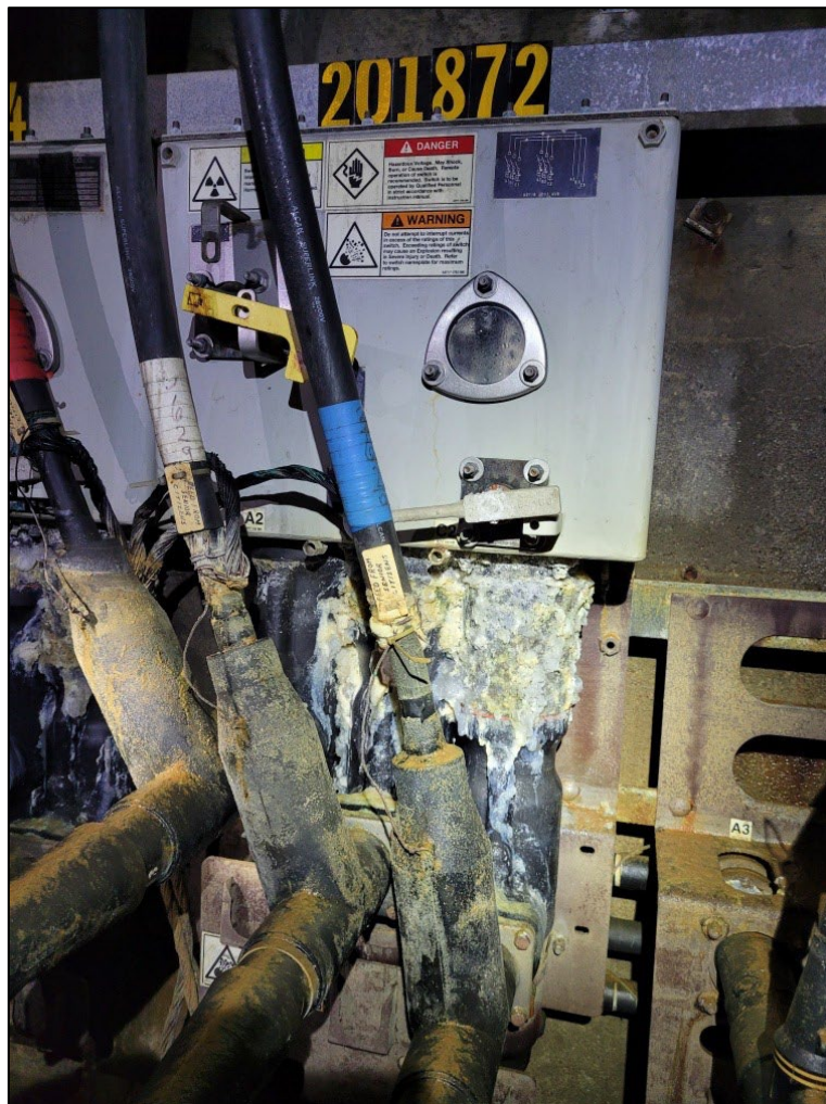
Figure 5.3.3 - 18 Corroded Submersible LBD Due to Flooding
