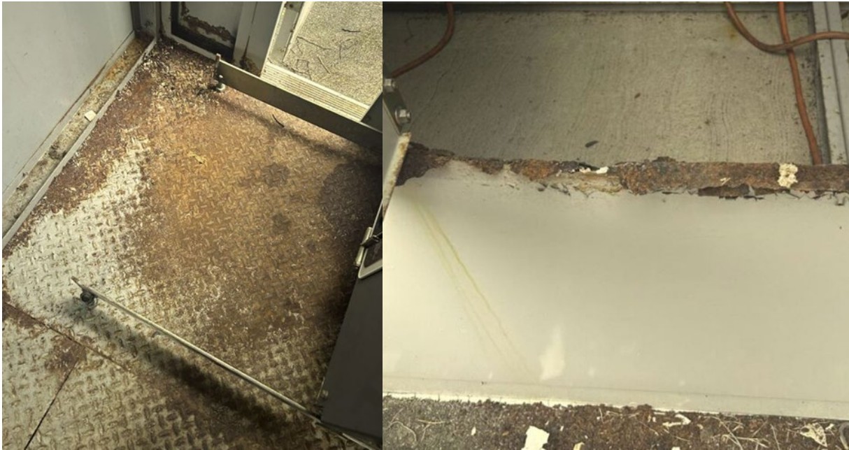
Figure 5.3.2 - 80 Rust inside a Station Switchgear Cabinet
