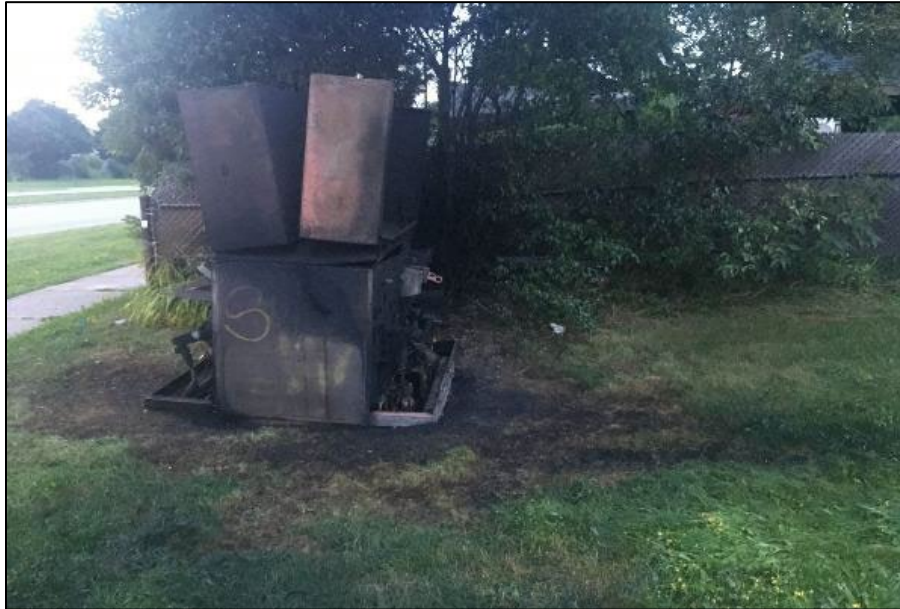
Figure 5.3.3 - 8 Failed Oil-Filled Switchgear
