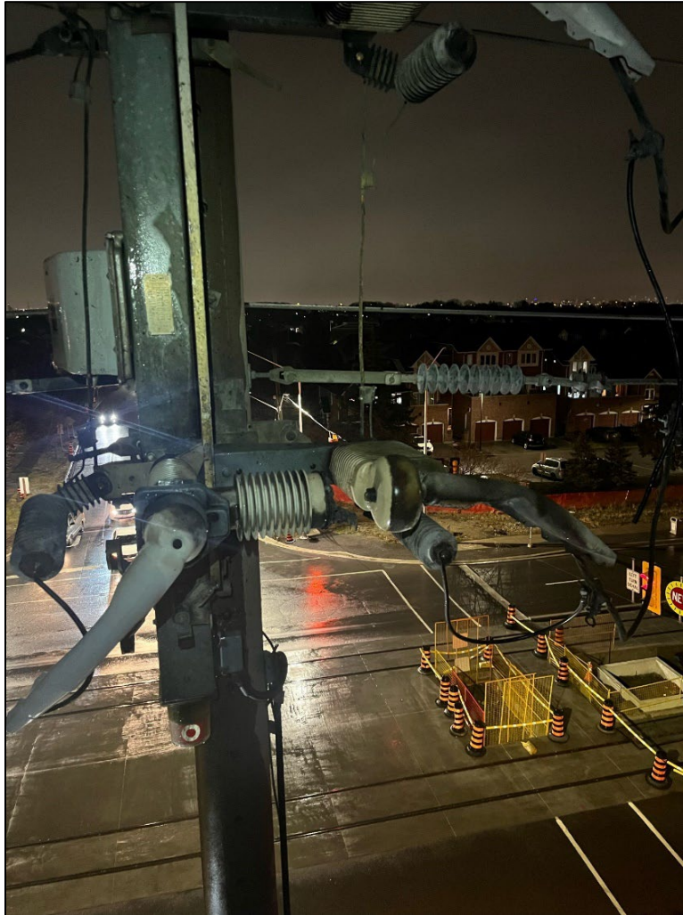
5 6 Figure 5.3.2 - 40 Mississauga – Flash Marks on Switch
