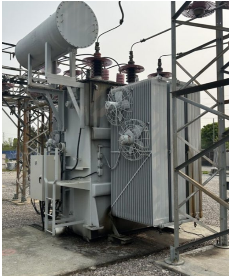
Figure 5.3.2 - 74 Power Transformer Experiencing an Oil Leak
