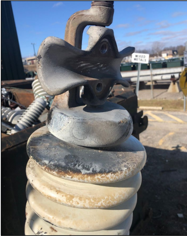
Figure 5.3.3 - 16 Pole Fire Due to Insulator Tracking
