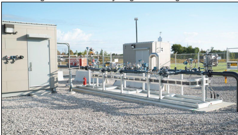
Figure 2: Markham Hydrogen Blending Station
