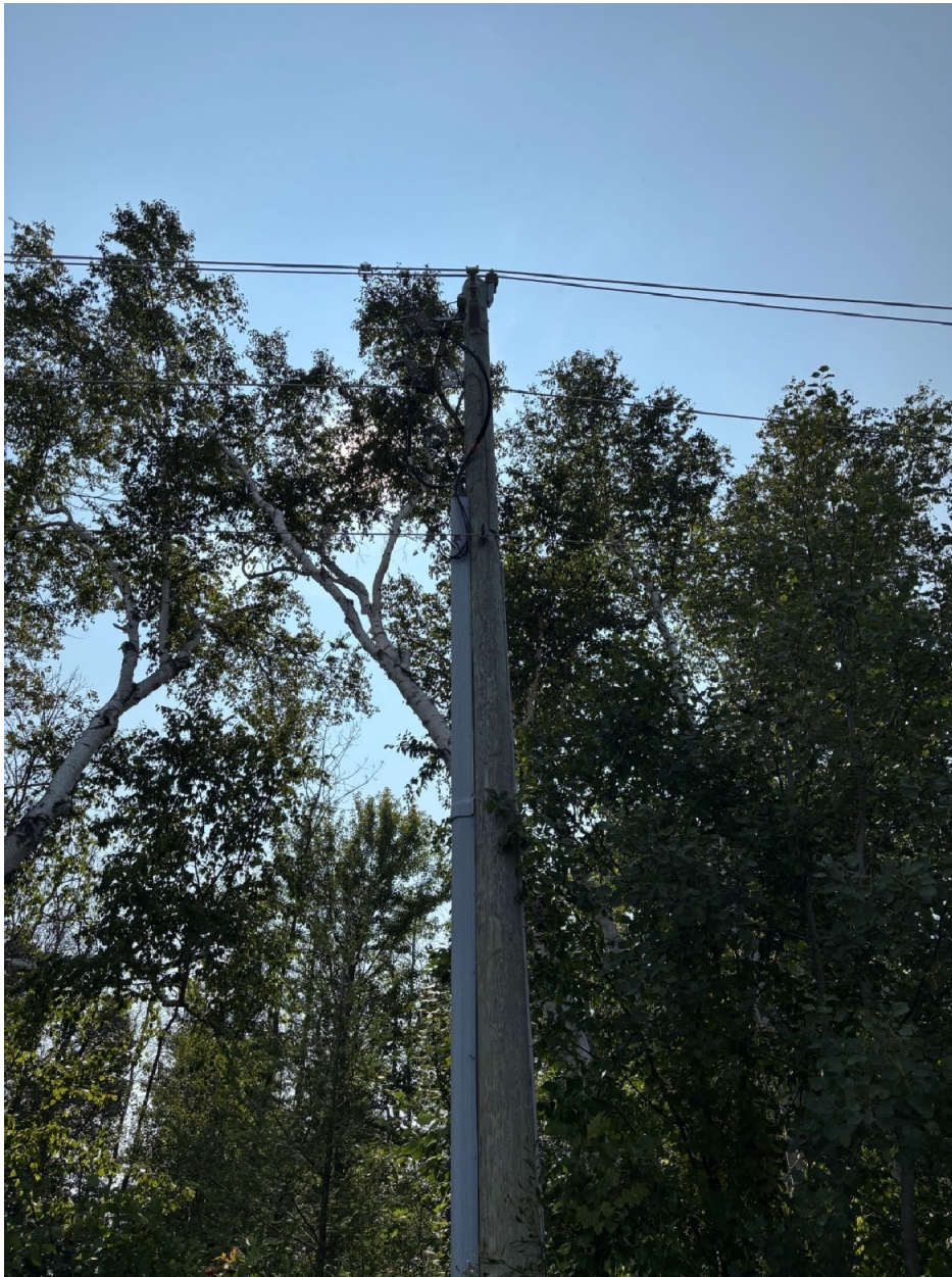
Picture #2: Three Phase Underground Dip
