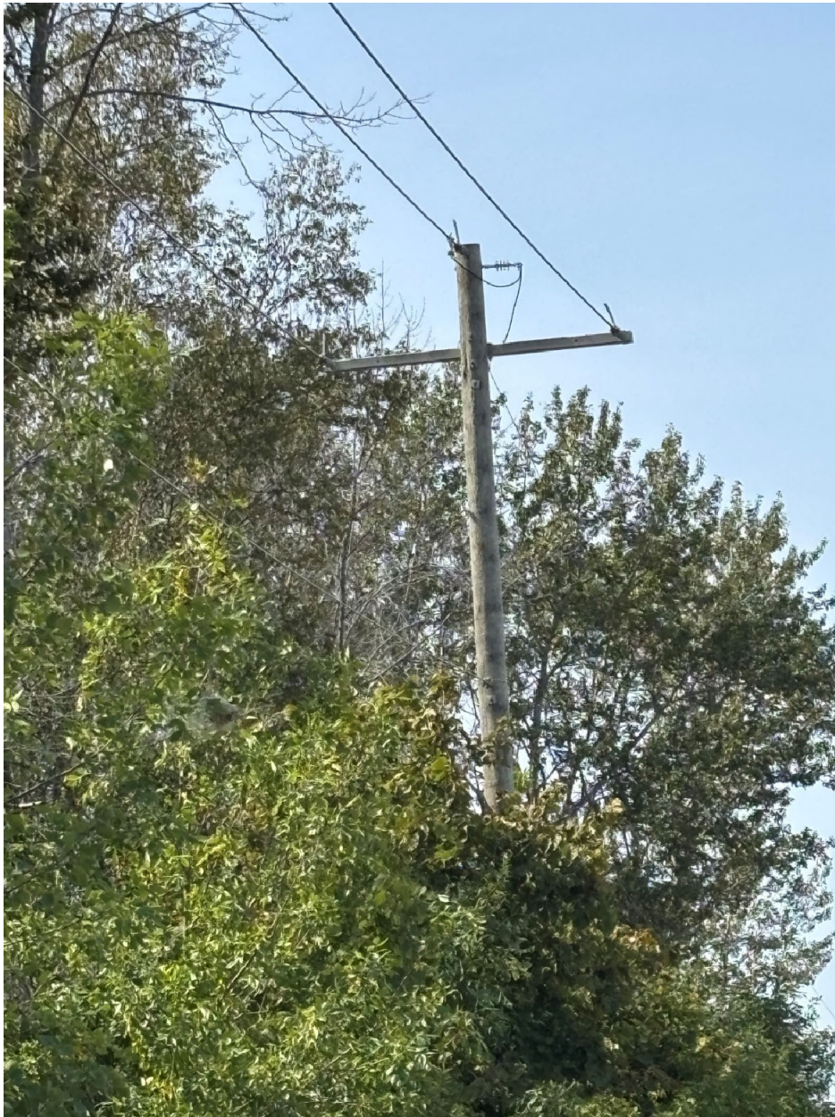
Picture #3: Three Phase WDI Dead-end
