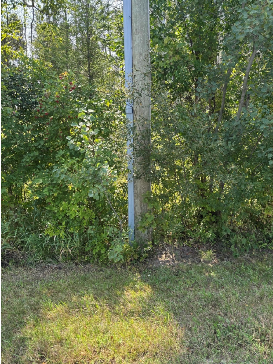
Picture #1: Three Phase Underground Dip
