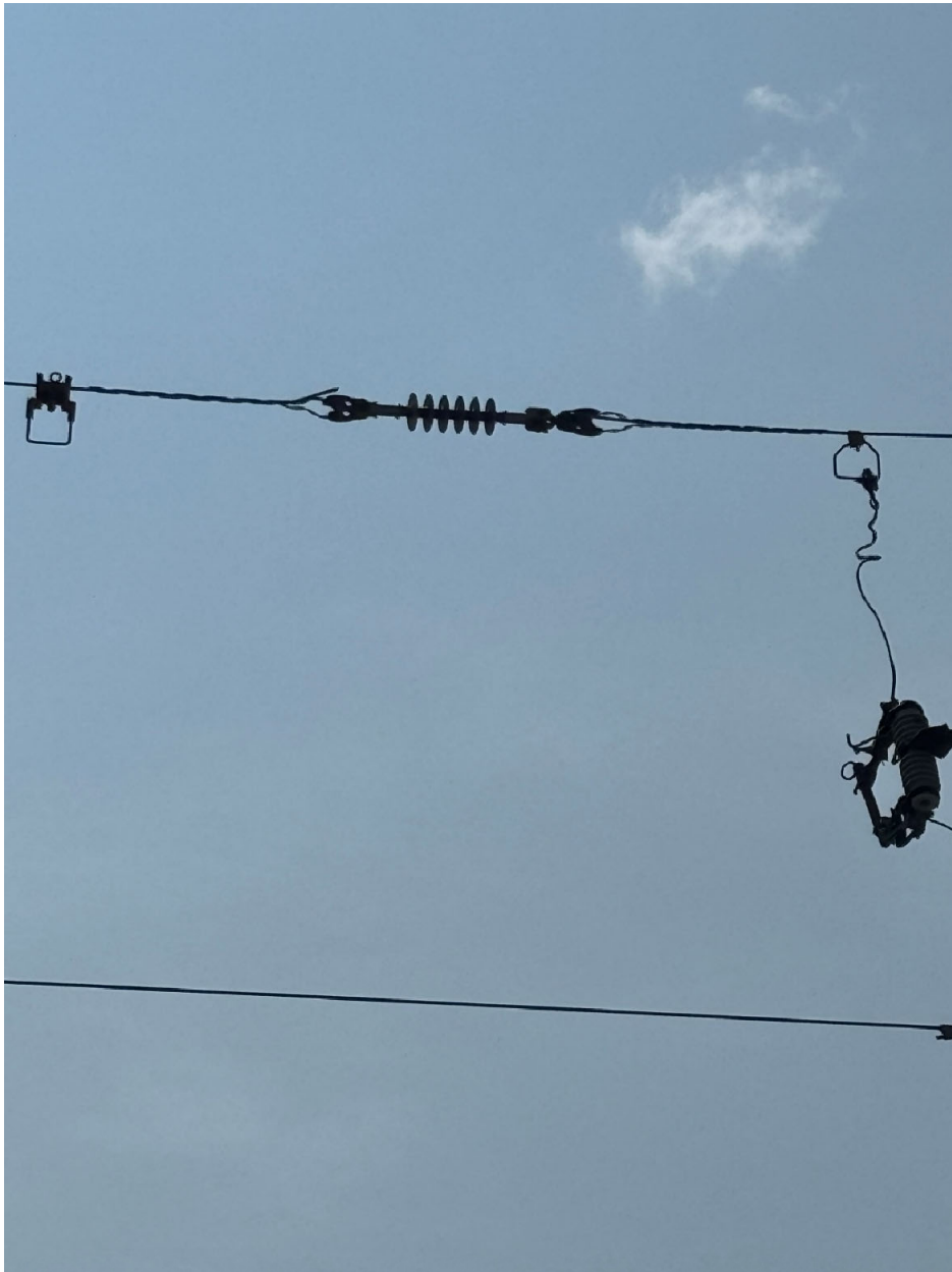
Picture #4: Hydro One Dead Span Open
