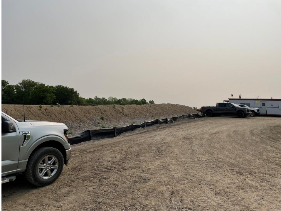
1. Temporary drilling pad, topsoil storage and silt fence (sediment and erosion control)
