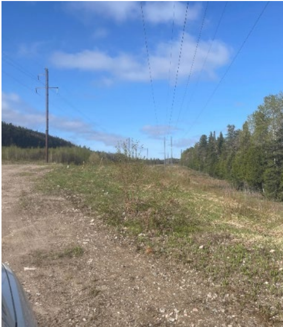
Photo 2: Examples of double pole groups for structural support at turns or longer spans
