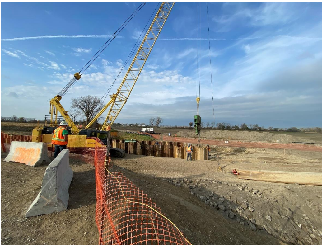
4. Sheet piling being utilized to stabilize the excavation near watercourse crossings with inconsistent soils.
