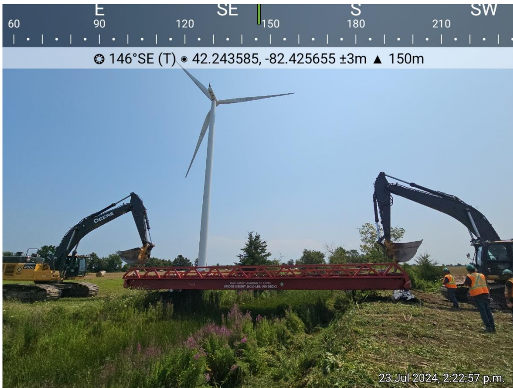
5. Clear span bridge being utilized to minimize environmental impact to this watercourse.
