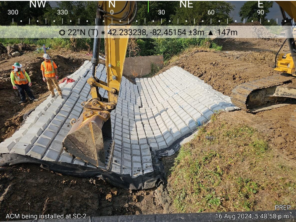
8. Watercourse restoration utilizing articulating cable concrete matting mandated by the Municipality of Lakeshore.
