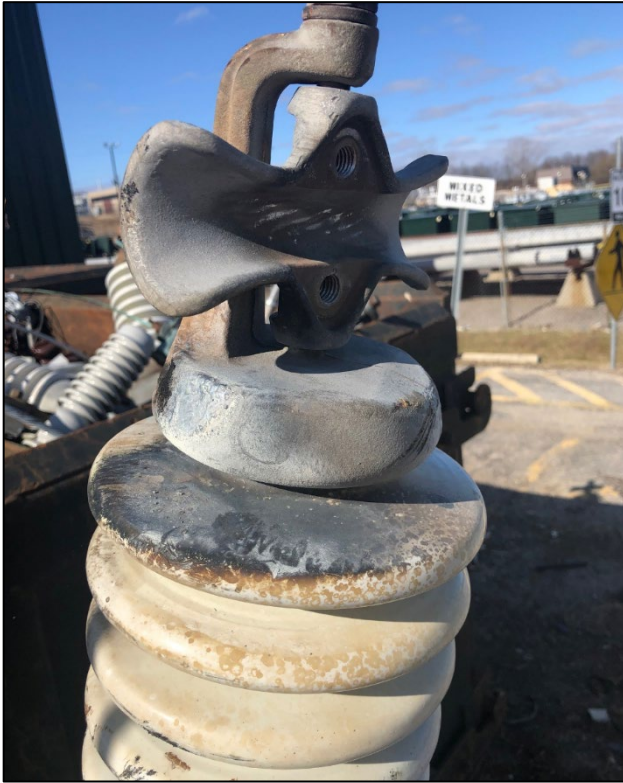
Figure 5.3.3 - 16 Pole Fire Due to Insulator Tracking
