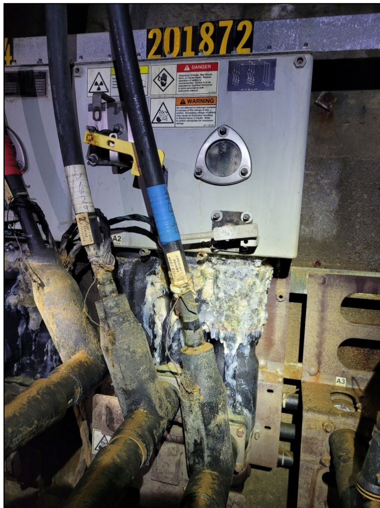
Figure 5.3.3 - 18 Corroded Submersible LBD Due to Flooding
