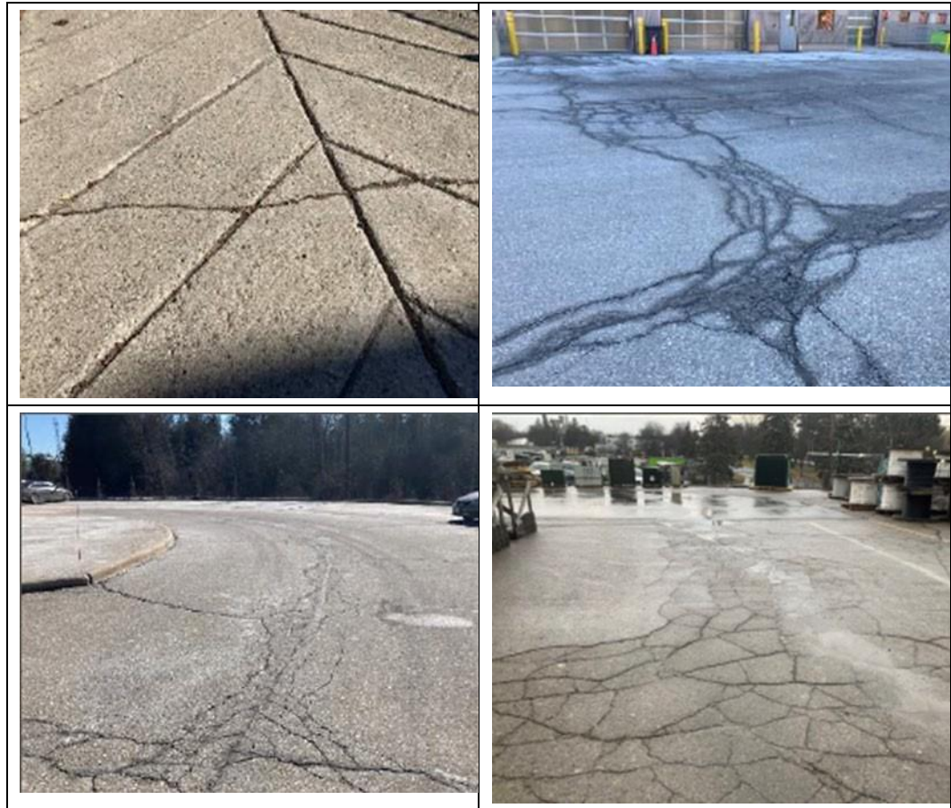
Figure B07 - 3 Examples of Outdoor Walkways/Driveways Deficiencies
