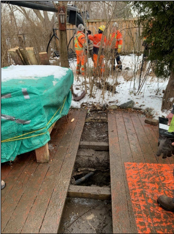
Figure 5.3.3 - 12 Cable Under Backyard Deck
