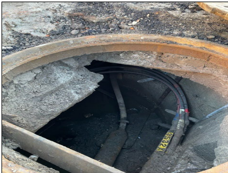
8 9 Figure 5.3.3 - 15 Hamilton – Cable Chamber Roof Collapse
