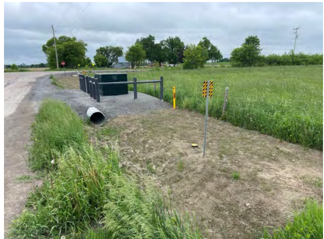
Photo 36: Restoration at the Enbridge Station located on Mcquinty Road near Snake River Line (June 9, 2025).
