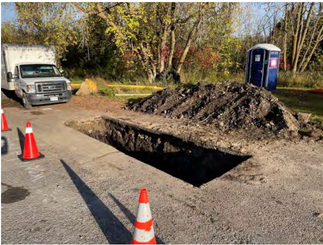
Photo 3: Tie-in pit within Micksburg Road shoulder, Tie-in was minimized in disturbance across the Project, where possible. (October 4, 2024).
