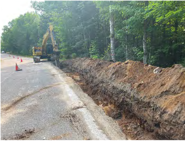
Photo 43: Existing conditions of open-cutting on southern shoulder of Mcgaghran Road (July 2, 2025).
