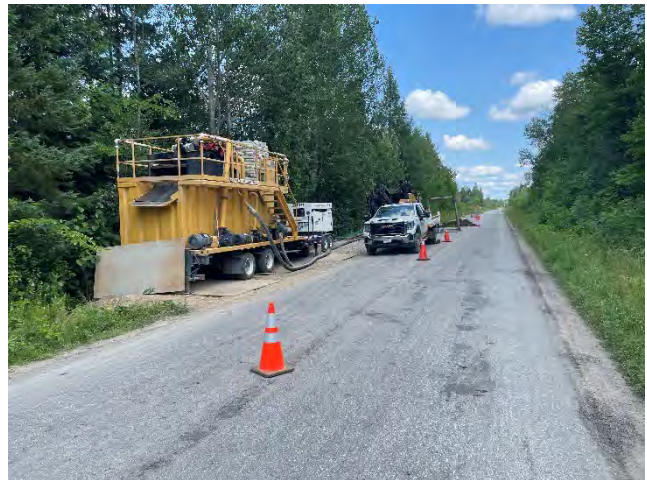
Photo 46: HDD drill rig staged and drilling on Cold Creek Road at Cold Creek (August 1, 2025).
