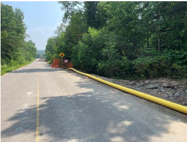
Photo 45: Existing conditions of pipeline prior to installation on Mcgaghran Road, west of Micksburg Road, east of Bulger Road (July 14, 2025).
