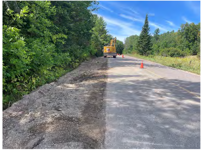
Photo 50: Backfilled and re-graded shoulder on Mcgaghran Road, east of Old Mine Road (August 29, 2025).
