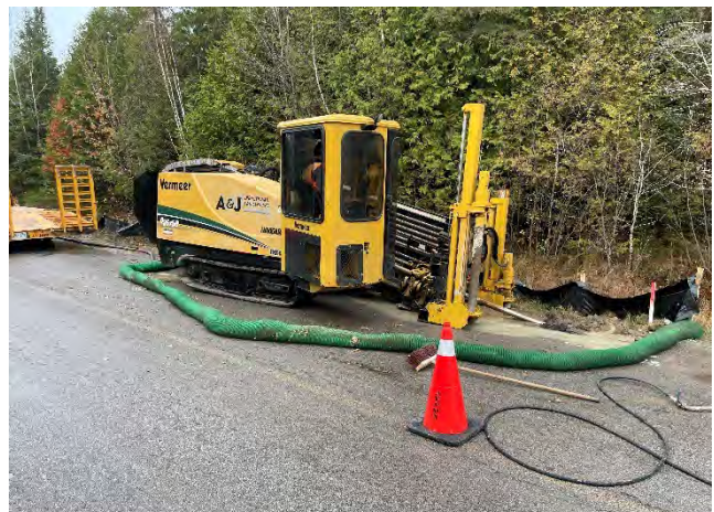
Photo 12: HDD drill rig staged and drilling within the Cold Creek Road ROW ditch. Silt sock established around drill rig during drilling to prevent off-site release of drilling mud (October 30, 2024).
