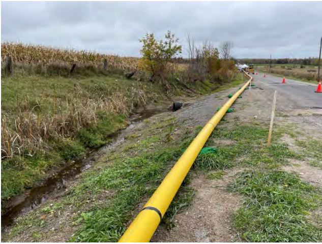
Photo 7: Pipeline stringing activities on Mcgaghran Road, near the watercourse crossing west of Pine Valley Road (October 15, 2024).
