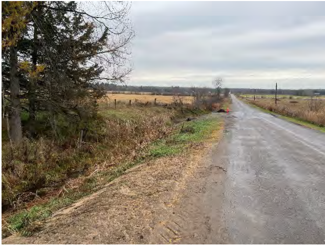
Photo 13: Backfilling completed at the entrance pit for the HDD crossing of the tributary to Snake River (November 4, 2024).
