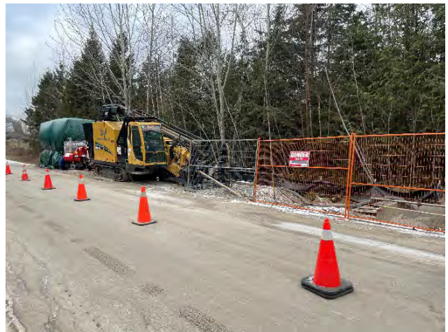
Photo 24: HDD drill rig staged and drilling within the Cold Creek Road ROW ditch (December 2, 2024).
