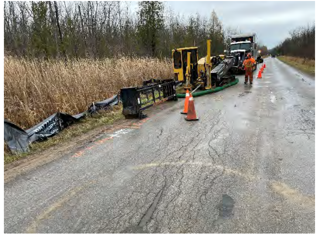
Photo 14: HDD drill rig staged and drilling within the Cold Creek Road ROW ditch in the Cold Creek wetland. (November 4, 2024).
