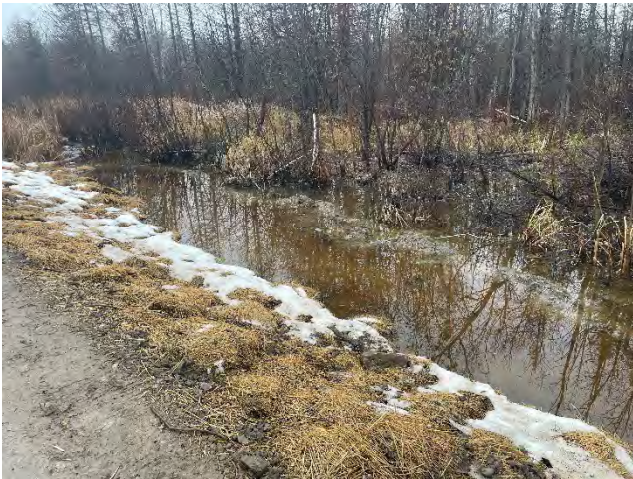
Photo 69: Existing conditions of strawbales spread to limit sedimentation into the ditch that flows into the Cold Creek watercourse (November 26, 2025).
