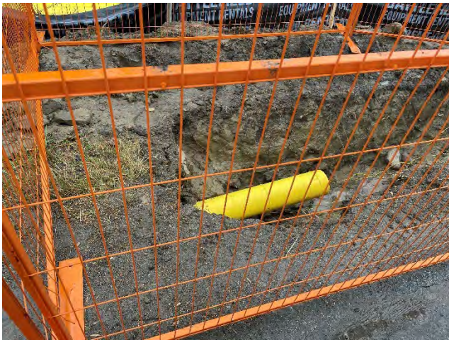
Photo 15: Tie-in pit within Cold Creek Road ROW ditch. Tie-in pits were minimized in disturbance where possible within the Cold Creek Wetland (November 4, 2024).
