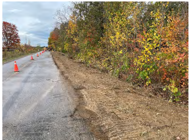
Photo 60: Restoration completed on Cold Creek Road, east of Mink Lake Road (October 10, 2025).
