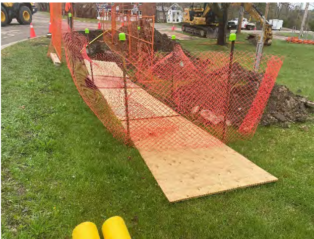
Photo 29: Existing conditions of tie-in location at the Bonnechere Street West and Mill Street intersection (May 9, 2025).
