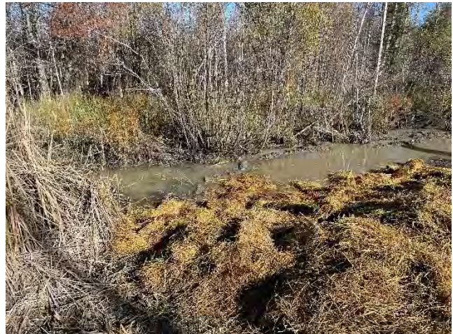
Photo 64: Existing conditions of strawbales spread to limit erosion of the ditch that flows into the Cold Creek watercourse (October 27, 2025).
