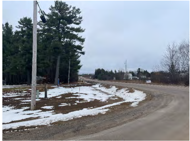
Photo 68: Completed restoration at corner of Cold Creek Road and Letts Cemetery Road (November 19, 2025).
