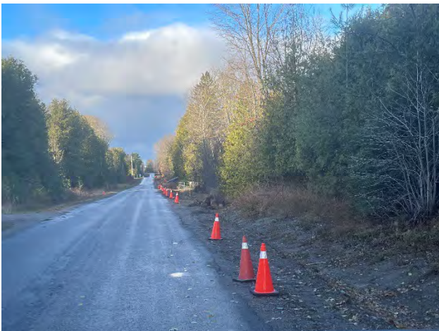
Photo 65: Restoration completed on Cold Creek Road, west of Mink Lake Road (November 6, 2025).
