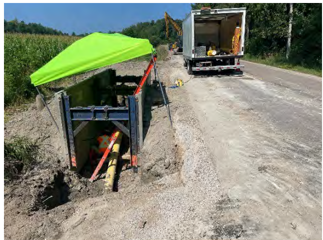
Photo 48: Existing conditions at tie-in on Mcgaghran Road, west of Old Mine Road (August 11, 2025).
