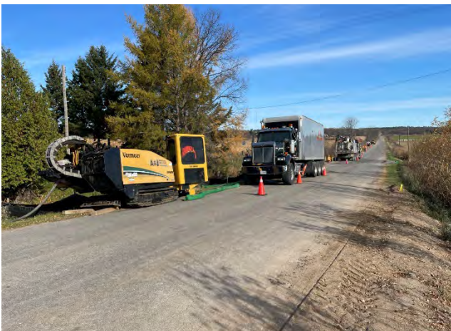
Photo 11: HDD drill rig staged and drilling within the Mcgaghran Road ROW ditch. Silt sock established around drill rig during drilling to prevent off-site release of drilling mud (October 30, 2024).
