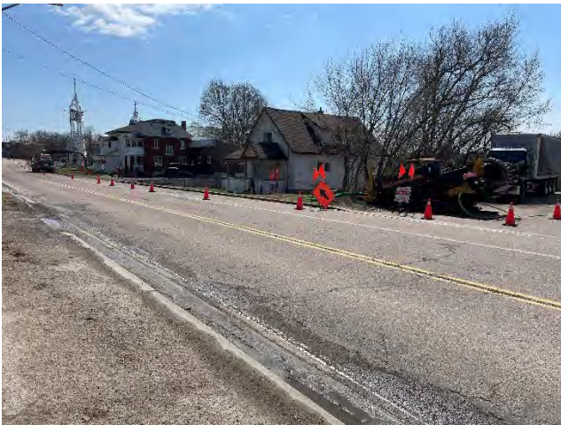
Photo 27: HDD drill rig staged and drilling within the Bonnechere Street West ROW near Bruce Street (April 24, 2025).
