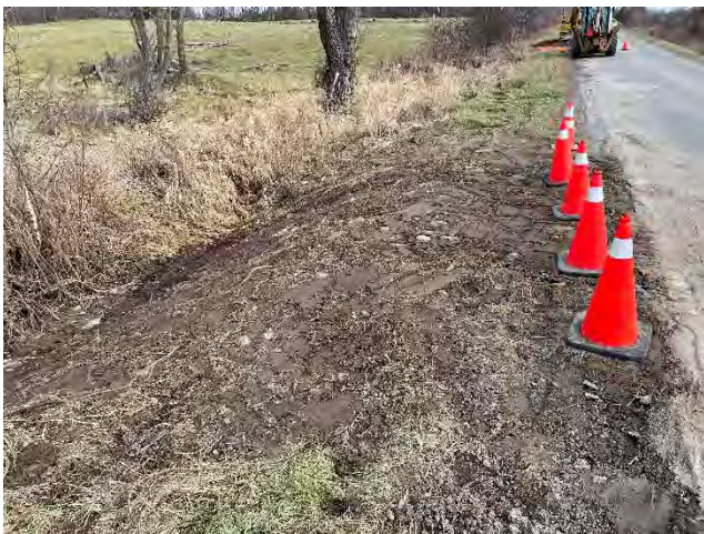
Photo 21: Restored tie-in location on Cold Creek Road, east of Mink Lake Road (November 25, 2024).
