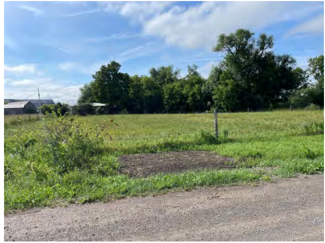
Photo 44: Backfilling completed at the entrance pit for the HDD crossing of the tributary to Snake River on Mcguinty Road (July 8, 2025).
