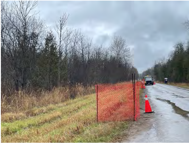
Photo 19: Existing conditions of daylighting hole during HDD drilling activities in the Cold Creek Wetland (November 11, 2024).
