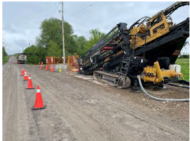
Photo 34: HDD drill rig staged and drilling on Mcquinty Road at tributary to Snake River (May 29, 2025).
