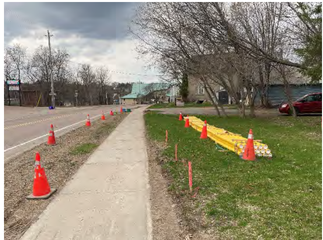
Photo 28: Existing conditions prior to pipeline stringing activities on Bonnechere Street East, facing west (May 5, 2025).
