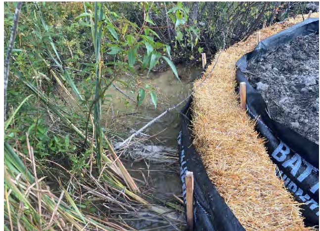
Photo 54: Sediment fencing and strawbales installed to prevent suspended sediment from entering Cold Creek, along the Cold Creek Road ROW (September 15, 2025)
