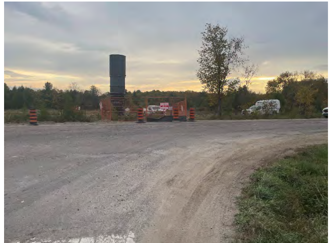
Photo 58: Energizing activities taking place at Bulger Road and Cold Creek Road intersection (October 10, 2025).
