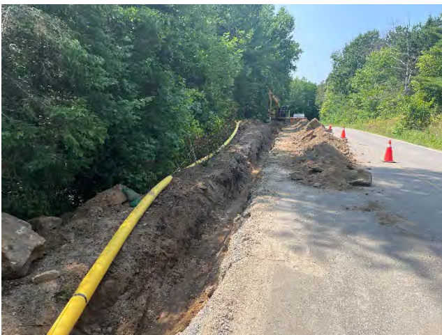
Photo 47: Existing conditions of pipeline prior to installation on Mcgaghran Road, west of Micksburg Road, east of Old Mine Road (August 8, 2025).
