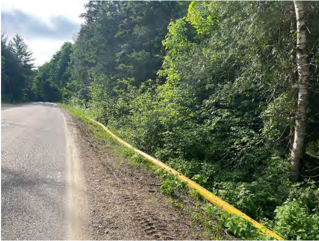
Photo 39: Existing conditions of pipeline prior to installation on Mcgaghran Road, west of Micksburg Road (June 22, 2025).
