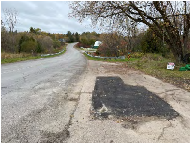
Photo 5: Remediation after tie-in was completed at same location as Photo 3. The tie-in pit was filled and re-surfaced with asphalt (October 15, 2024).
