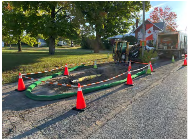
Photo 4: HDD location on Micksburg Road. Silt sock established around drill rig during drilling to prevent off-site release of drilling mud (October 4, 2024).
