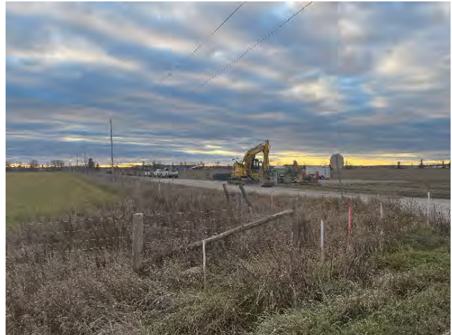
Photo 20: Existing conditions of Enbridge Station Work at McGuinty Road and Snake River Line, facing northwest. (November 18, 2024).
