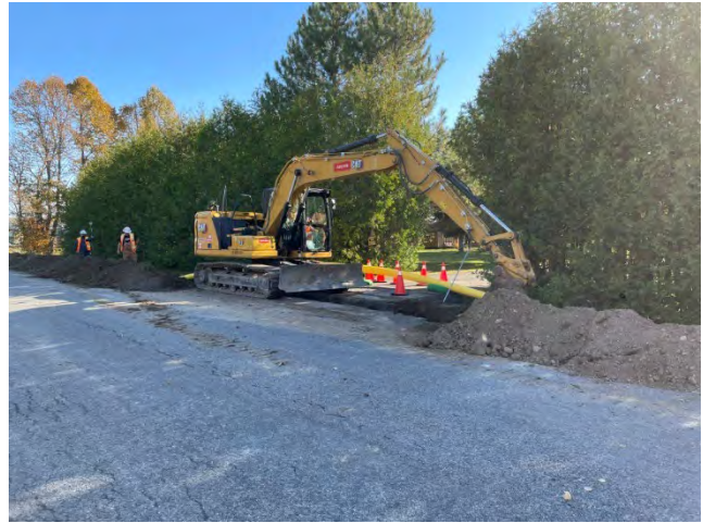
Photo 8: Excavation activities where pipeline stringing occurred on Mcgaghran Road, east of Bulger Road (October 21, 2024).
