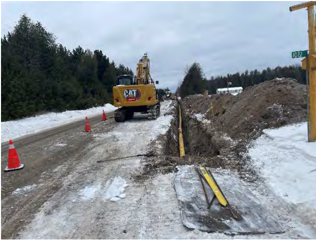
Photo 25: Mainline pipeline strung along road embankment on Cold Creek Road ROW (December 9, 2024).
