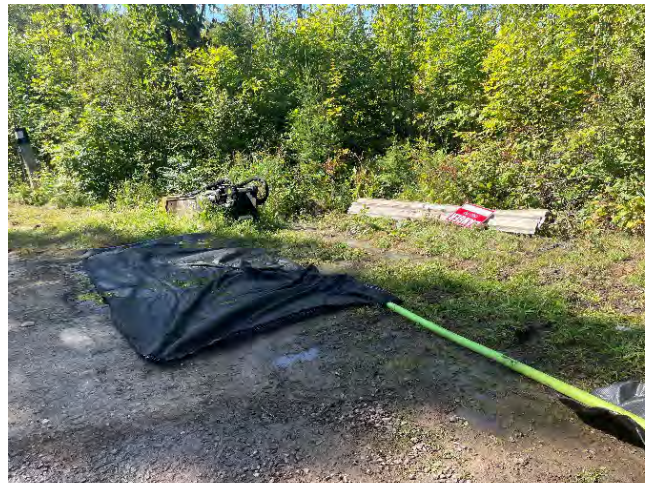
Photo 52: Established de-watering location through a filter bag at shoring box location on Cold Creek Road (September 5, 2025).
