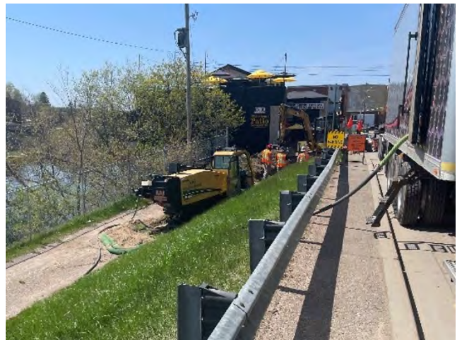
Photo 30: HDD drill rig staged and drilling on the ROW of Bonnechere Street West. Silt sock established around drill rig during drilling to prevent off-site release of drilling mud (May 13, 2025).
