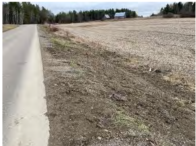
Photo 22: Restored road embankment on MCGAGHRAN ROAD between Bulger Road and Old Mine Road (November 28, 2024).
