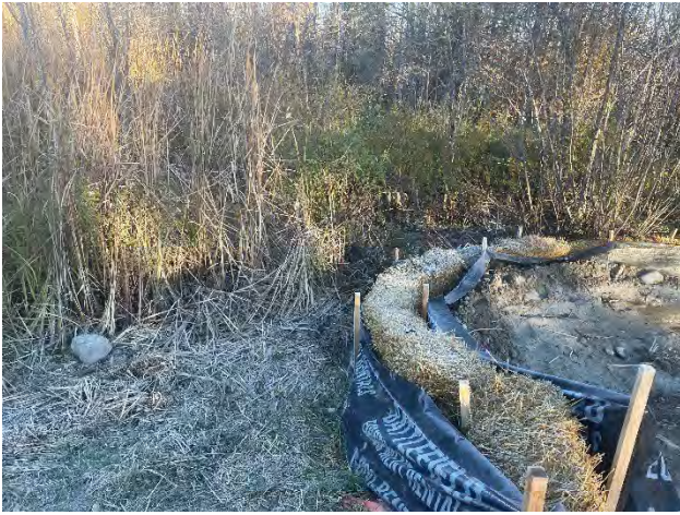
Photo 61: Existing conditions of ESC control at shoring box location within Cold Creek wetland (October 17, 2025).
