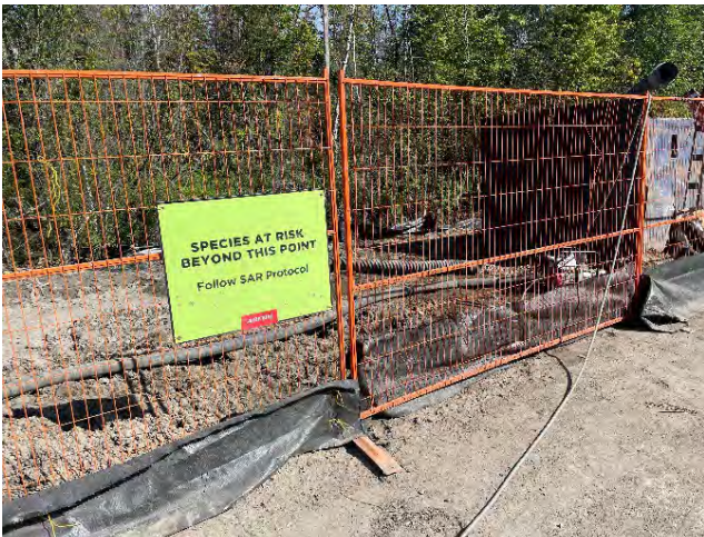
Photo 51: Existing conditions at shoring box location to assist HDD drilling activities within Cold Creek Wetland, east of Cold Creek (September 5, 2025).
