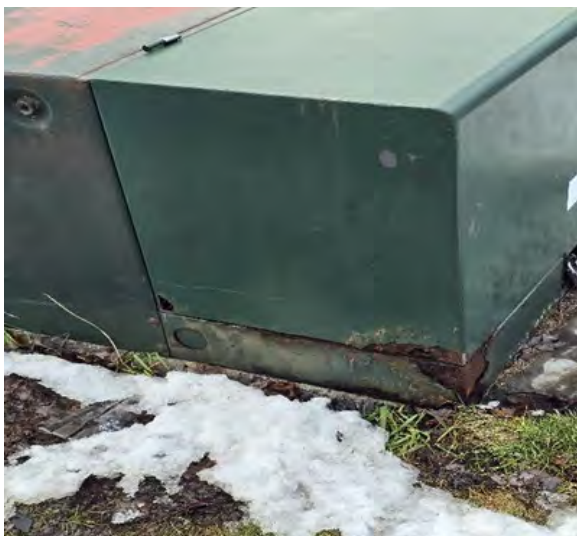
Figure 5: Rusted Padmount Transformer
