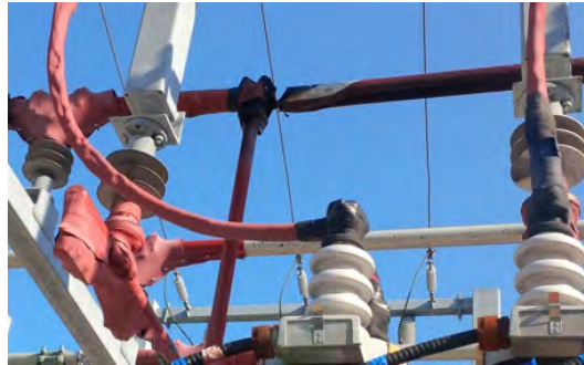
1 Figure 9: Bus work failure at Bay Ridges Substation
