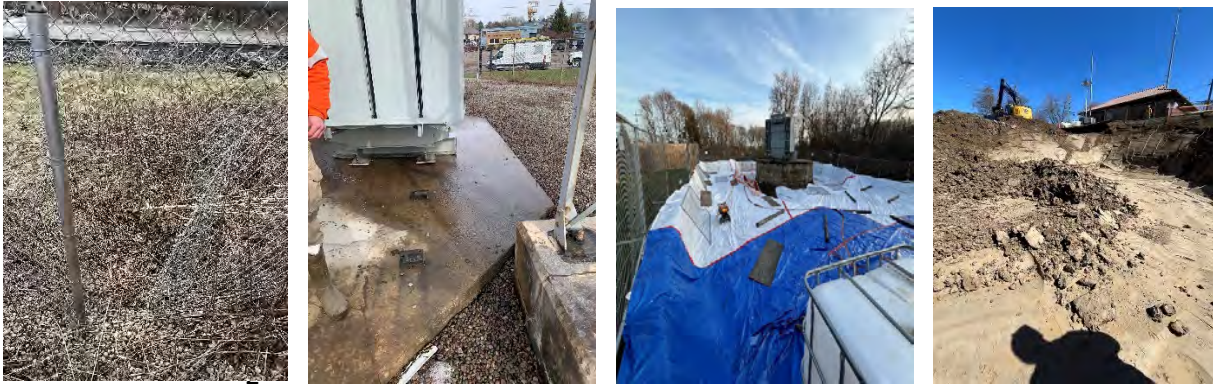
1 Figure 10: 2024 Substation Vandalism Incident
