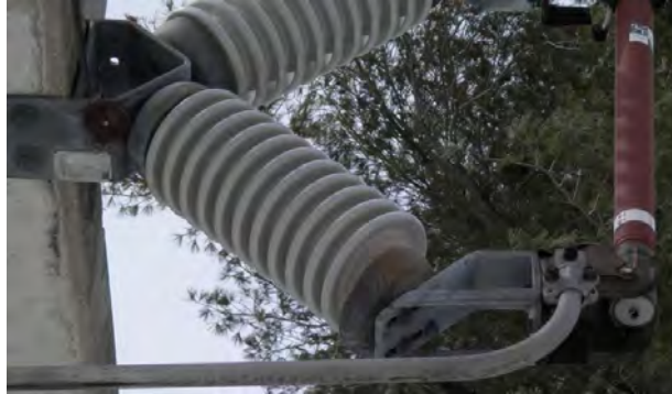
1 Figure 8: Broken Insulator at First Substation
