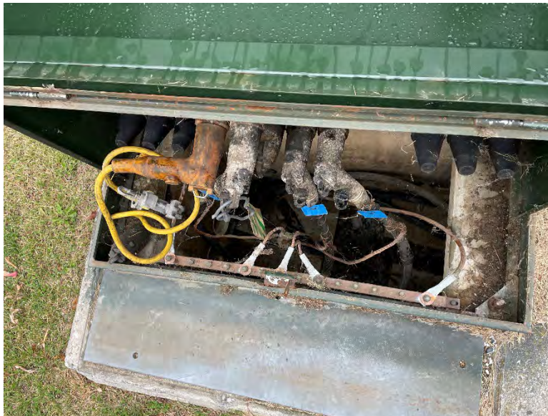
Figure 7: Severely Corroded Elbows on Padmount Switchgear Termination
