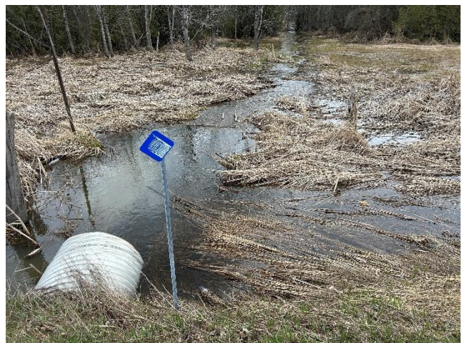
Photo 12: Water flowing through regulated watercourse on Sanford Road where the ditchwater from Photo 11 enters the watercourse (April 14, 2026).
