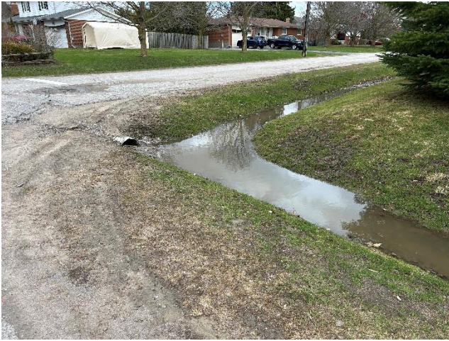
Photo 25: Water ponding at the corner of Smith Drive and James Place in spring 2026 in the Village of Sanford from clogged culverts and poor drainage, see Photo 26 (April 14, 2026).
