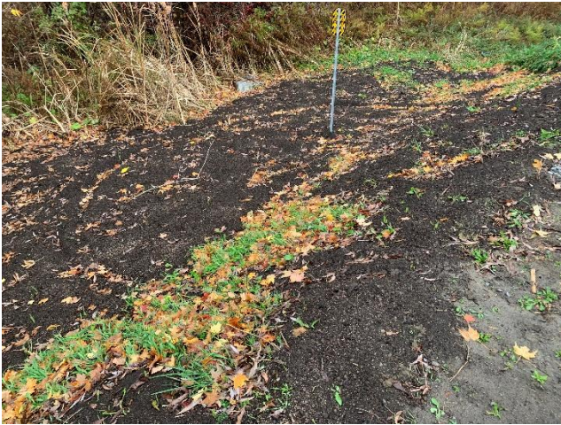
Photo 5: Restoration completed in CA regulated area at the corner of Ball Road and Centre Road at the conclusion of construction in 2024 (October 10, 2024).
