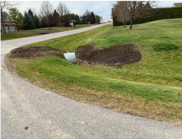
Photo 27: Reclaimed road ditch along Lundy Drive after the completion of construction (November 14, 2024).
