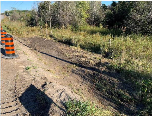
Photo 15: Backfilling completed at the entrance pit for the HDD crossing of Leaksdale Creek after the completion of construction in 2024 (September 26, 2024).
