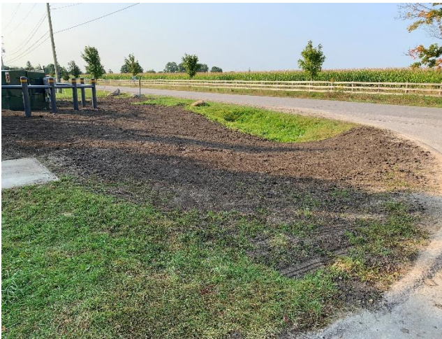
Photo 3: Restoration completed around the upgraded station at the southeast Corner of Bolton Road and Concession 6 at the conclusion of construction (September 13, 2024).
