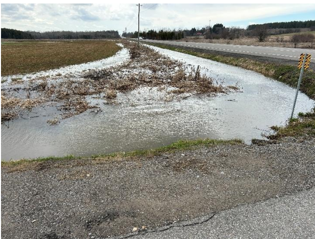
Photo 11: Water flowing through ditch at the reclaimed southwest corner of Bolton Road and Concession 6 (April 14, 2026).
