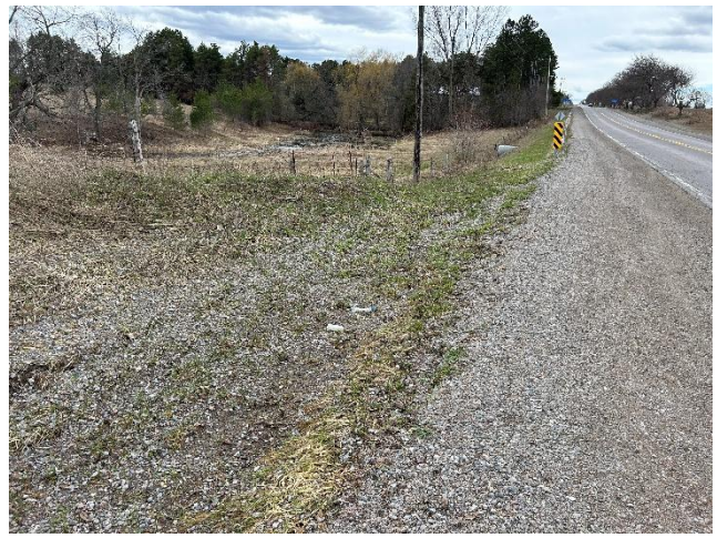
Photo 22: Restored road embankment east of the Village of Sanford on Sandford Road at the location from Photo 21 (April 14, 2026).
