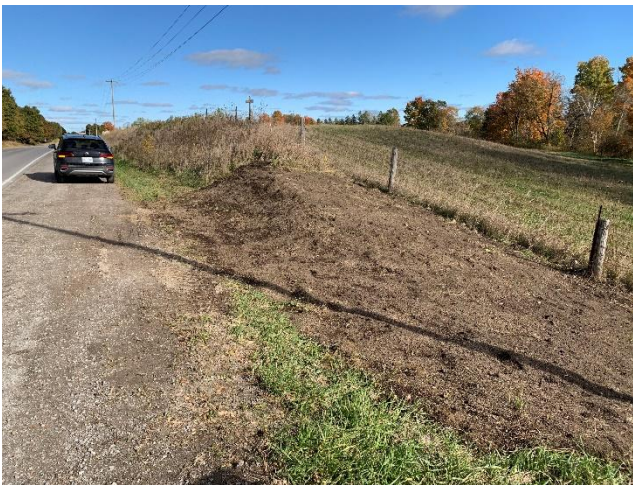
Photo 21: Restored road embankment east of the Village of Sanford on Sandford Road after the completion of construction (October 16, 2024).
