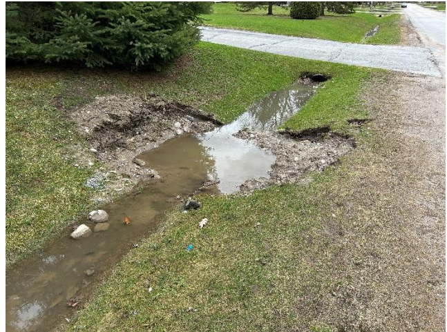
Photo 26: Water ponding and clogged culverts down gradient of the corner of Smith Drive and James Place constraining natural flow, not the result of project activities (April 14, 2026).
