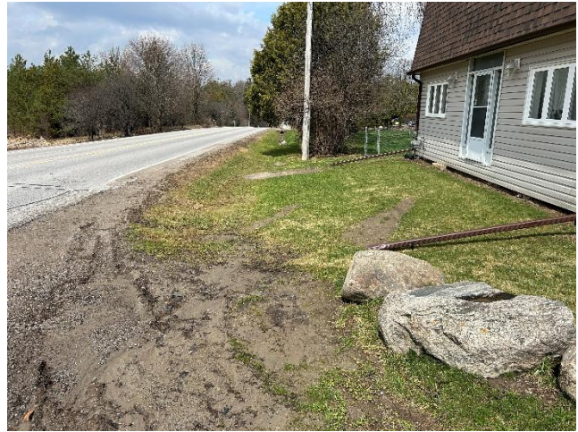
Photo 20: Restored road embankment in spring 2026 on Photo 19. Winter road maintenance appears to deposit large amounts of sand on lawn on the corner of Concession 6 and Davis Drive (April 14, 2026).
