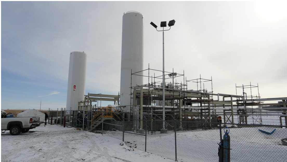
14 TPD Liquefaction Plant
